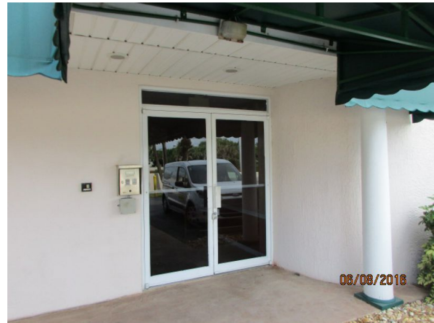
Unprotected Glazed Entry Door
