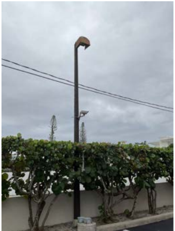
Parking lot lights (6)
