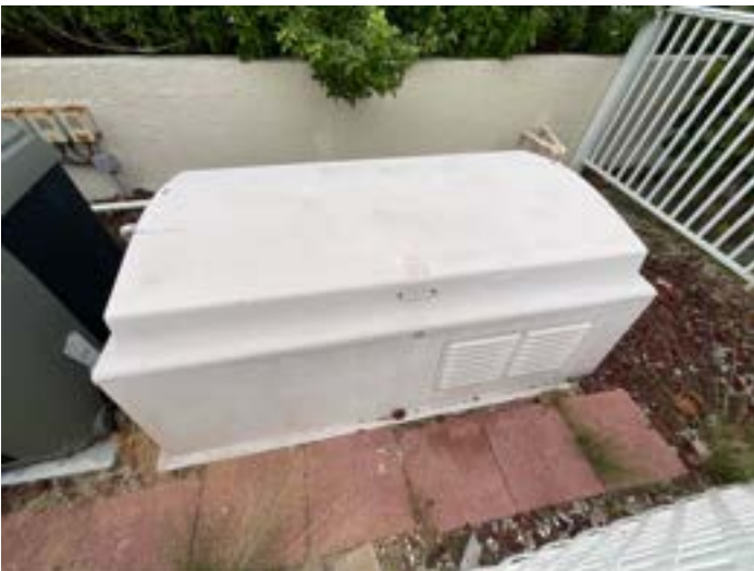
Pool equipment - 2 total
