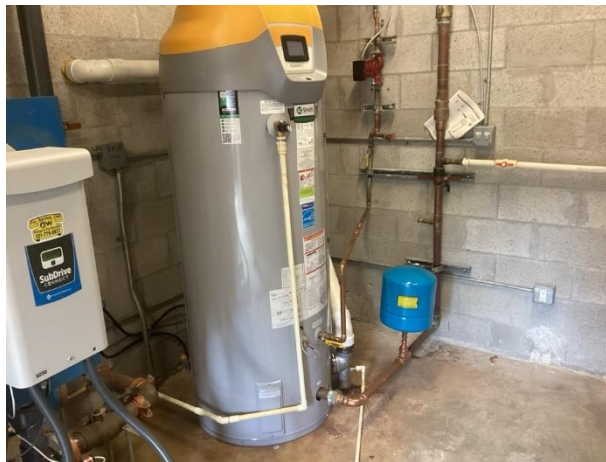
Domestic water boiler
