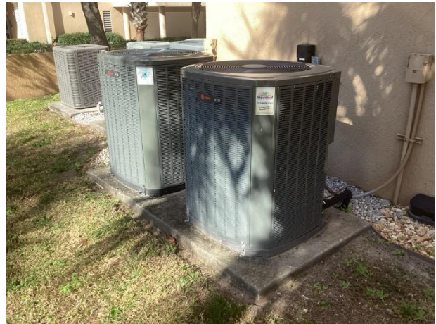
Split system condensing units
