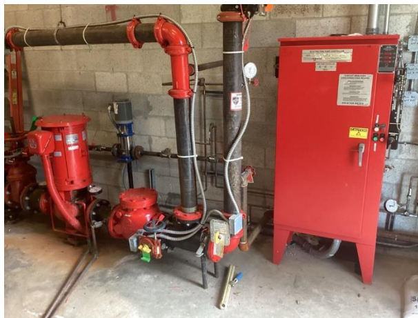
Fire suppression pump
