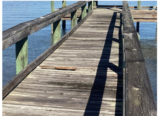
Deck board damage
