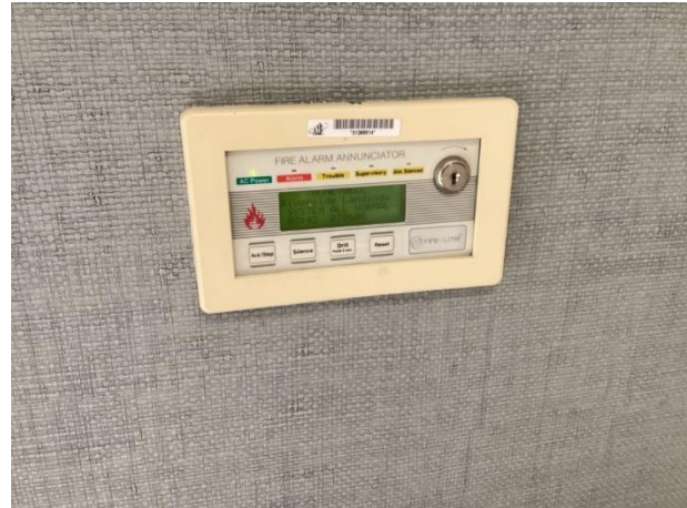
Secondary control panel
