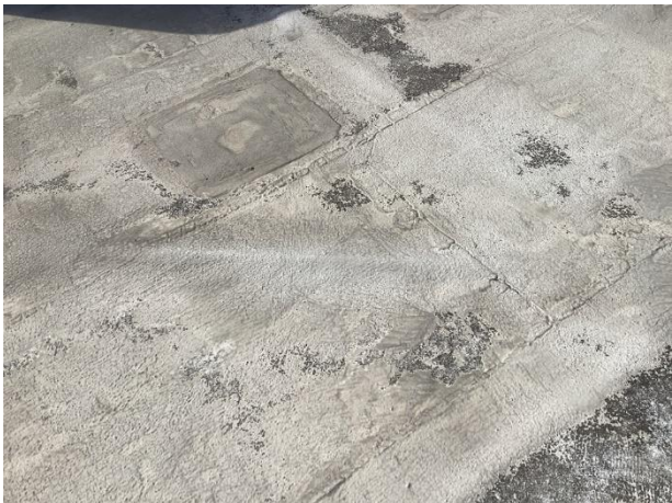
Bulges in the membrane
