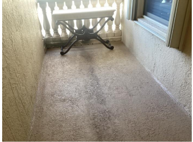
Coating deterioration at the concrete breezeways
