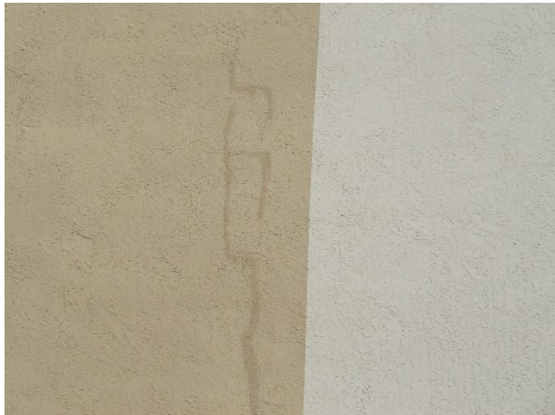
Evidence of previously repaired cracks
