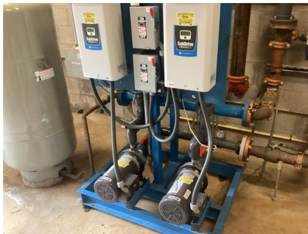
Domestic water pumps
