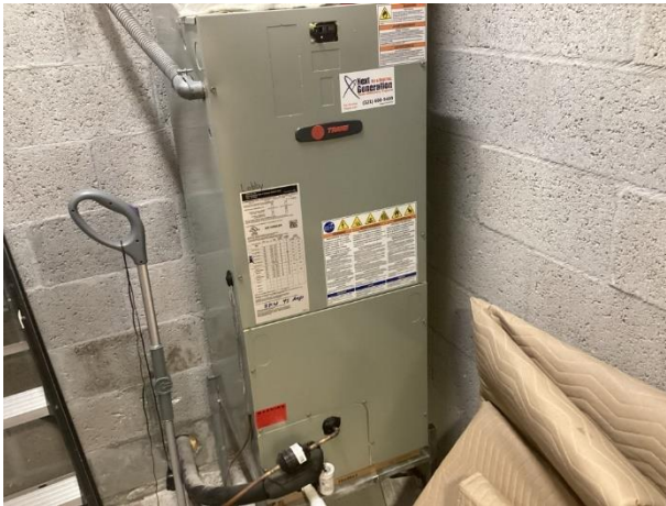
Split system air handling unit
