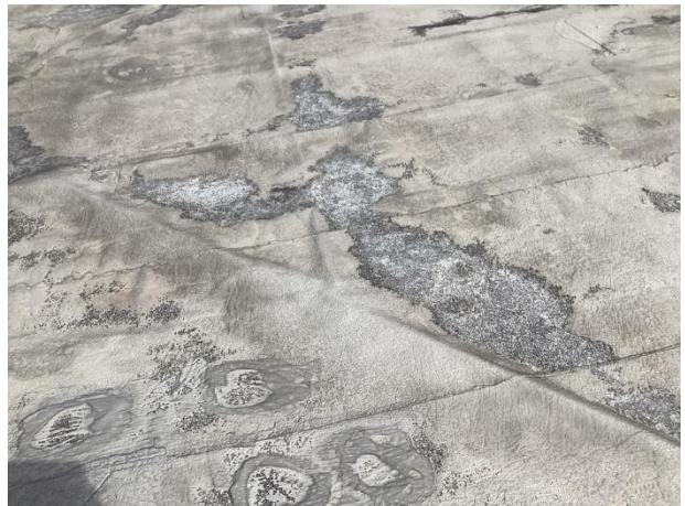
Bulges in the membrane
