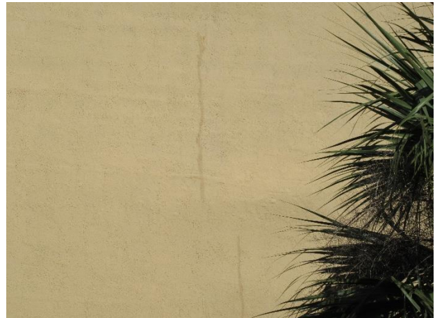
Evidence of previously repaired cracks
