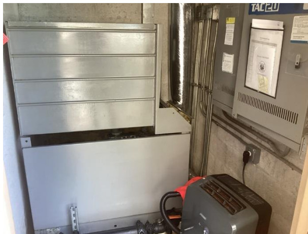
Hydraulic elevator equipment
