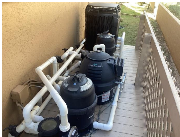
Pool mechanical equipment
