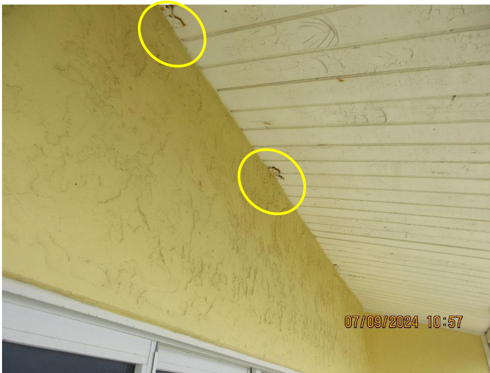
View of corroded hurricane straps
