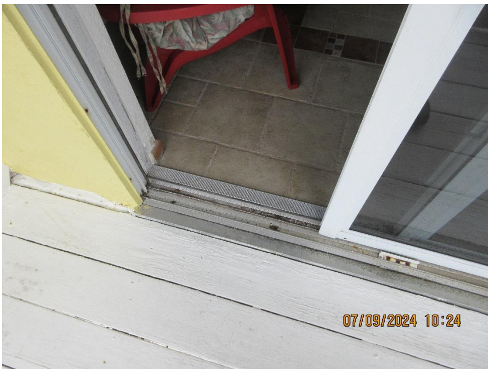
View of corroding sliding glass door fasteners
