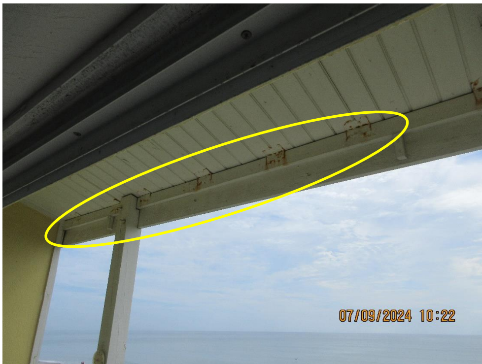
View of corroded hurricane straps
