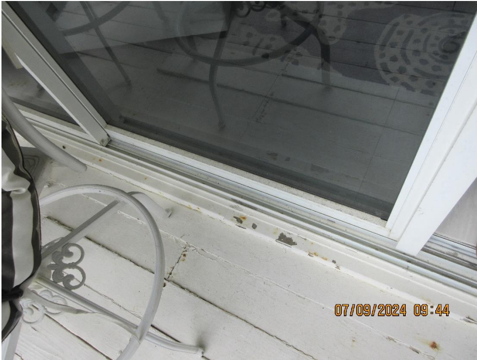
View of corroding sliding glass door track
