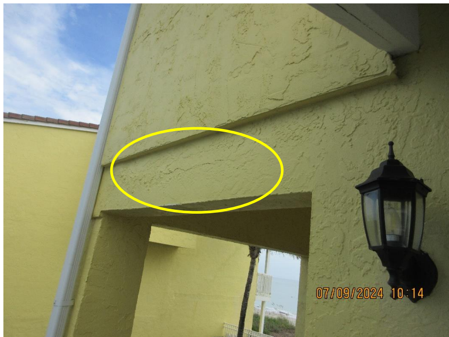
View of stucco crack near unit entryway
