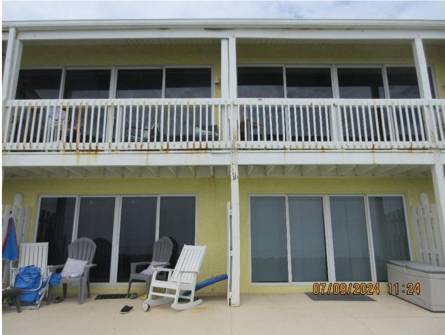
View of staining caused by corrosion of non-stainless-steel fasteners
