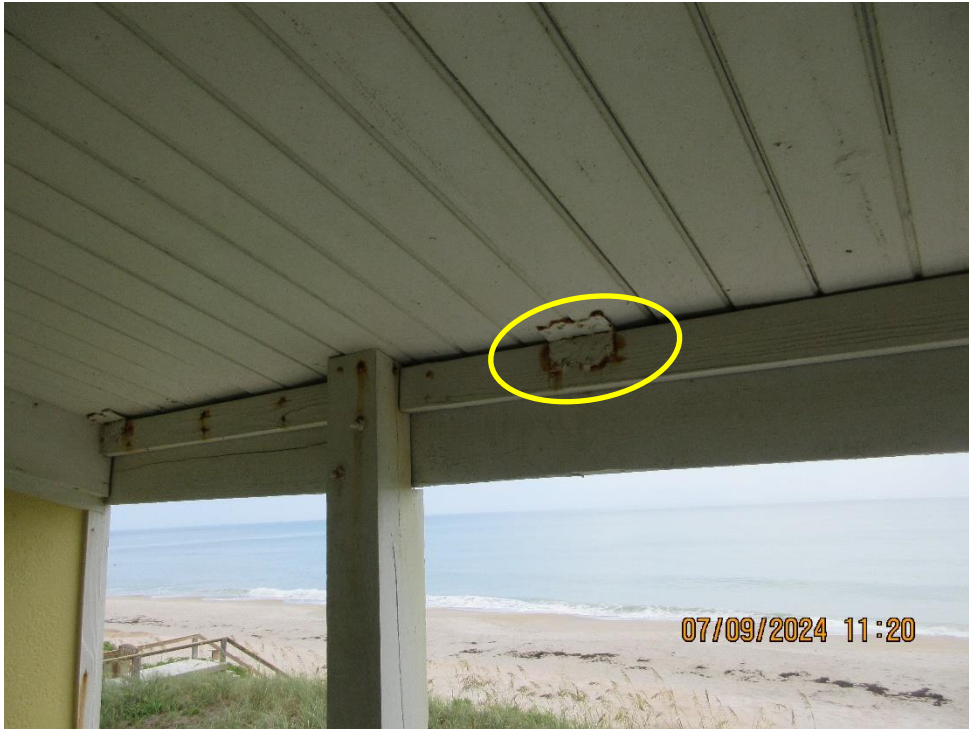
View of corroded hurricane strap and fasteners
