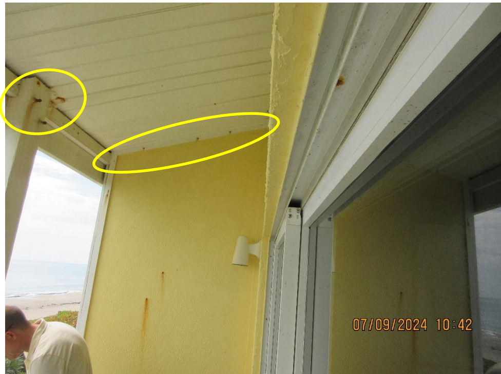
View of corroded fasteners
