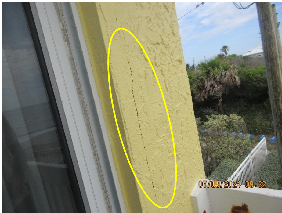
View of stucco cracks near sliding glass door
