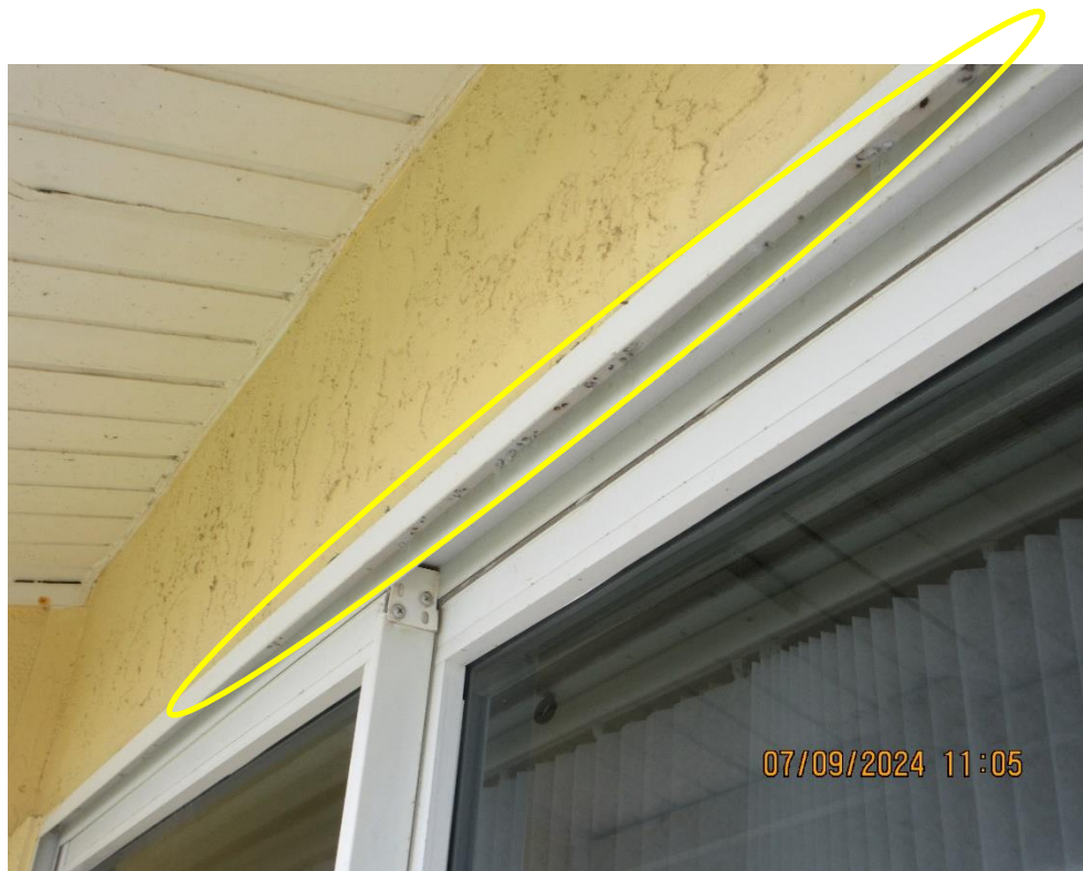
View of corroding sliding glass door track
