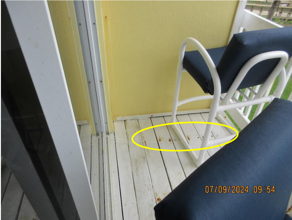
View of corroded deck fasteners
