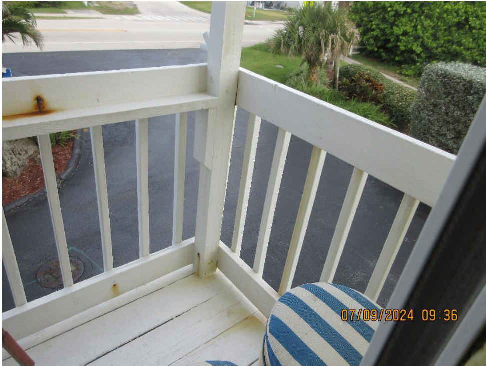
View of corroded railing fasteners
