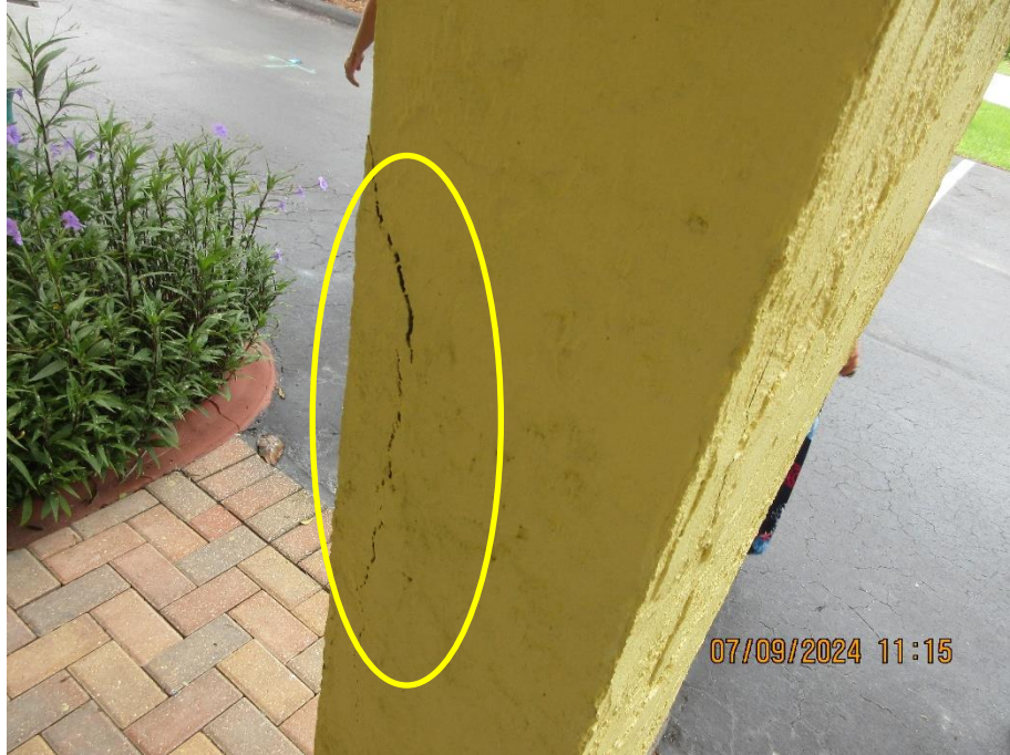
View of stucco crack in west elevation column
