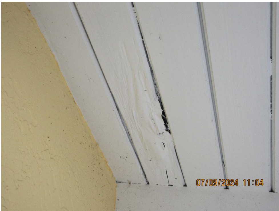
View of deteriorated ceiling board
