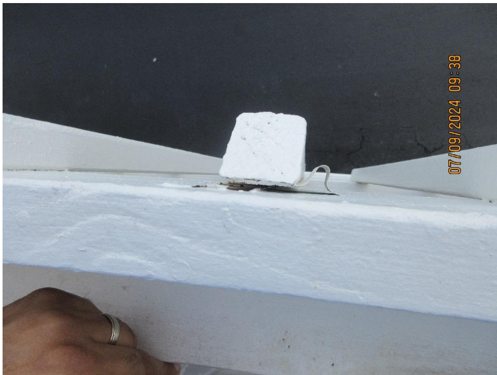
View of loose railing picket.
