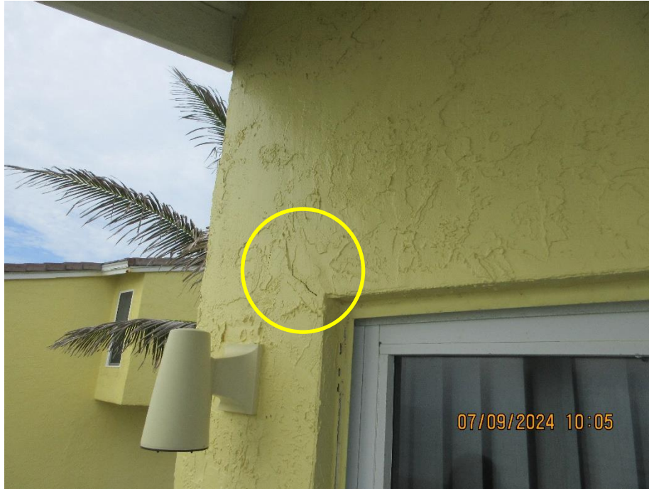
View of stucco crack near balcony sliding glass door
