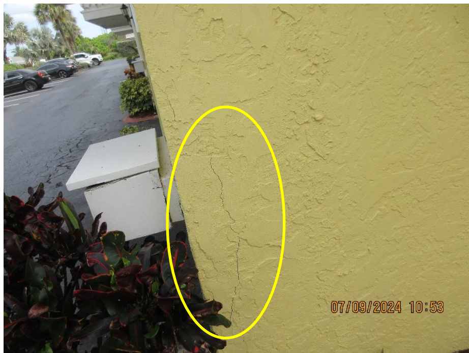
View of stucco crack at unit entryway
