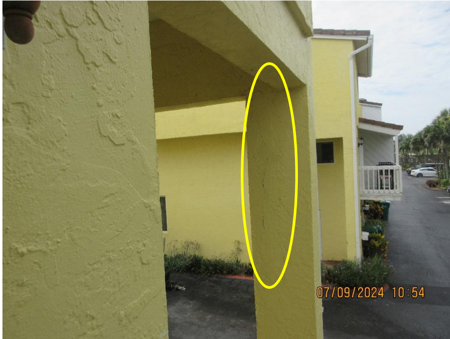
View of stucco crack above unit entryway
