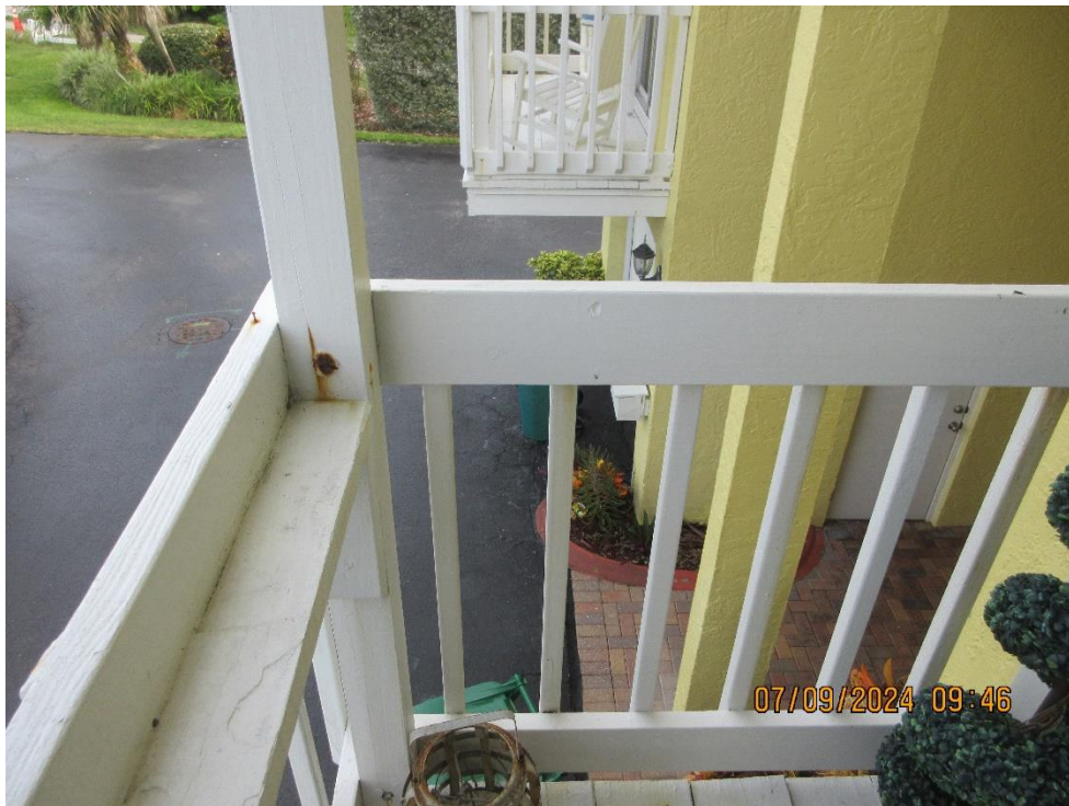
View of corroded railing fasteners
