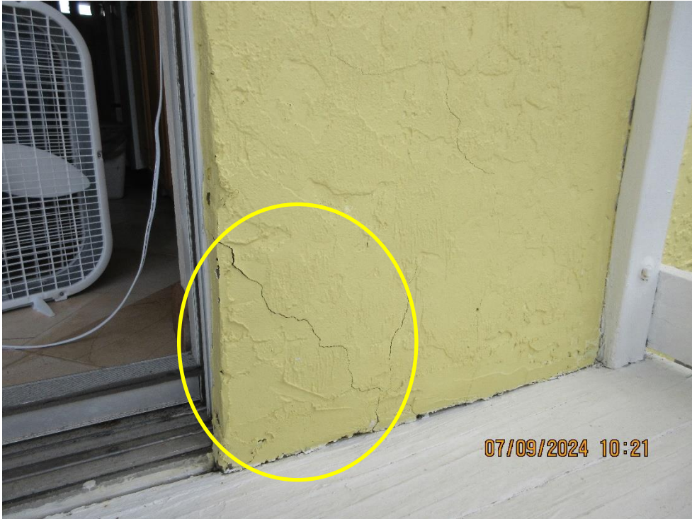
View of stucco crack near sliding glass door
