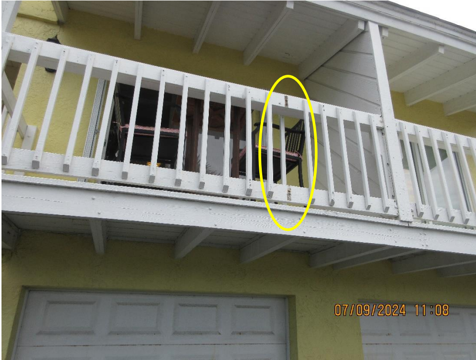
View of loose/missing railing picket
