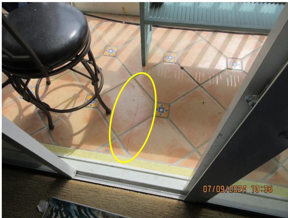
View of tile installed over the original balcony structure. Note crack in tile
