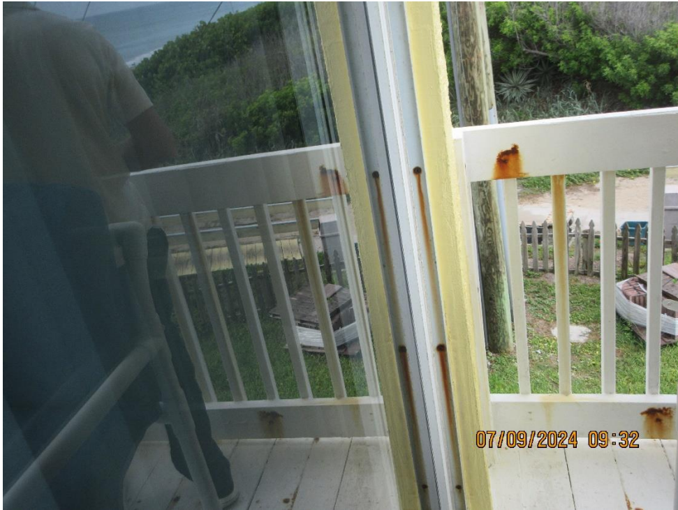
View of corroding sliding glass door fasteners
