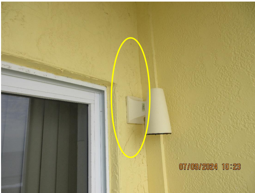
View of stucco crack at light fixture
