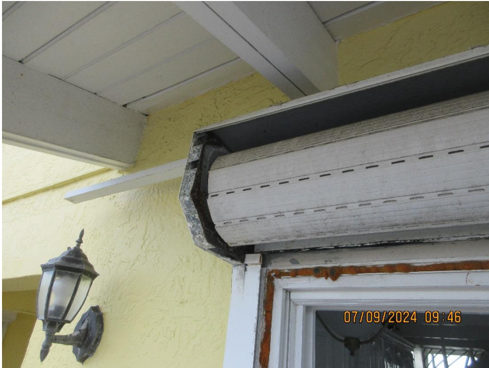
View of missing shutter box cover and Styrofoam sealant
