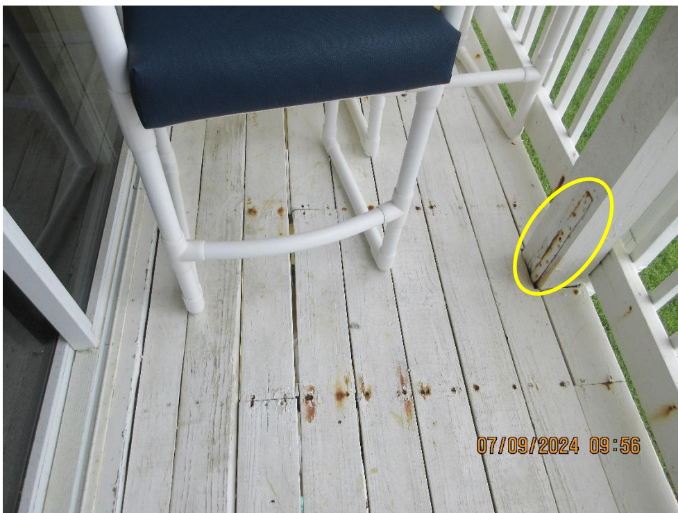
View of corroded hurricane strap and deck fasteners
