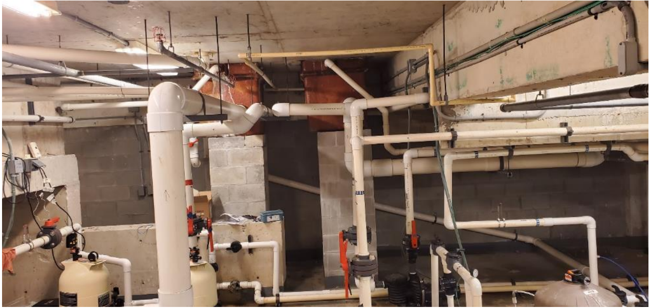
View of pool pump room (3 rd Floor)
