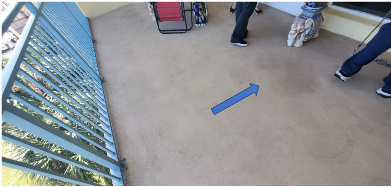
Evidence of ponding water on the balcony surface. (Unit 407) Could be improved during a future restoration project
