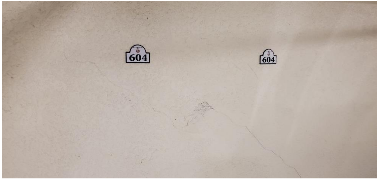
Concrete wall in garage with cracks and spalls Repair cracks and repaint, monitor for potential future concrete repair
