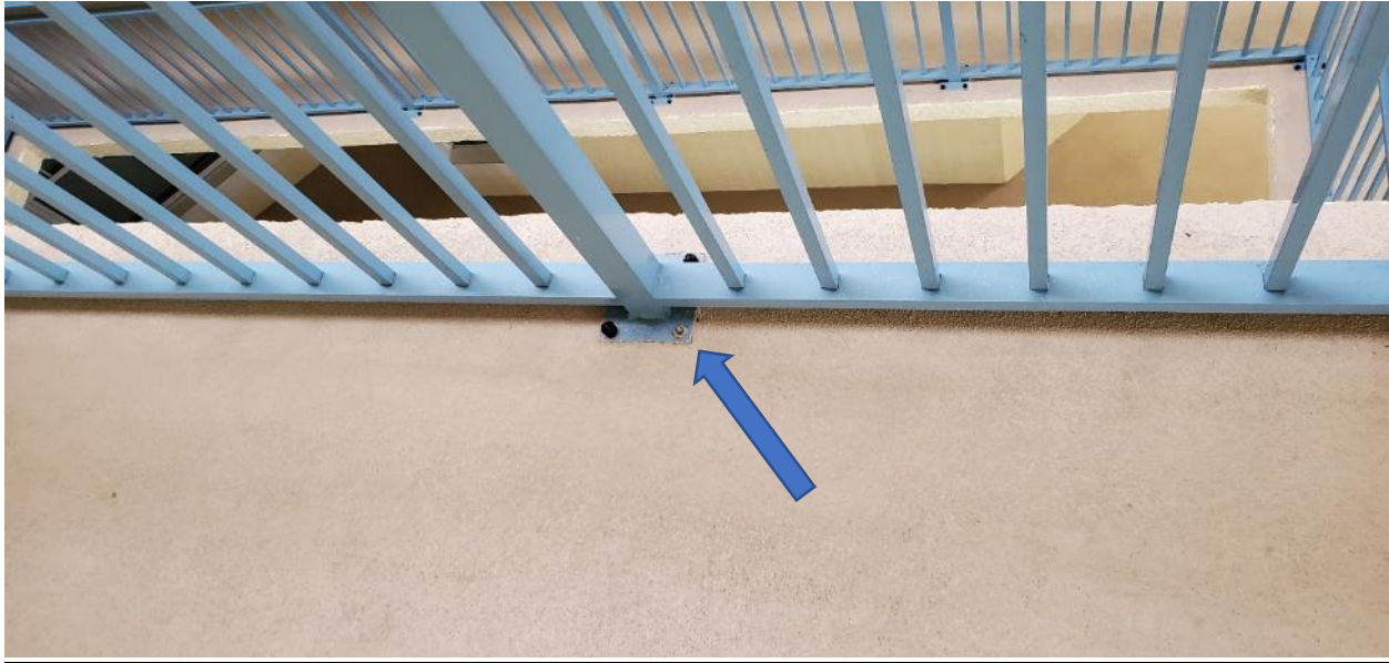
Missing fastener cap on walkway railing (7 th Floor) Consider repainting railings during next building painting project.
