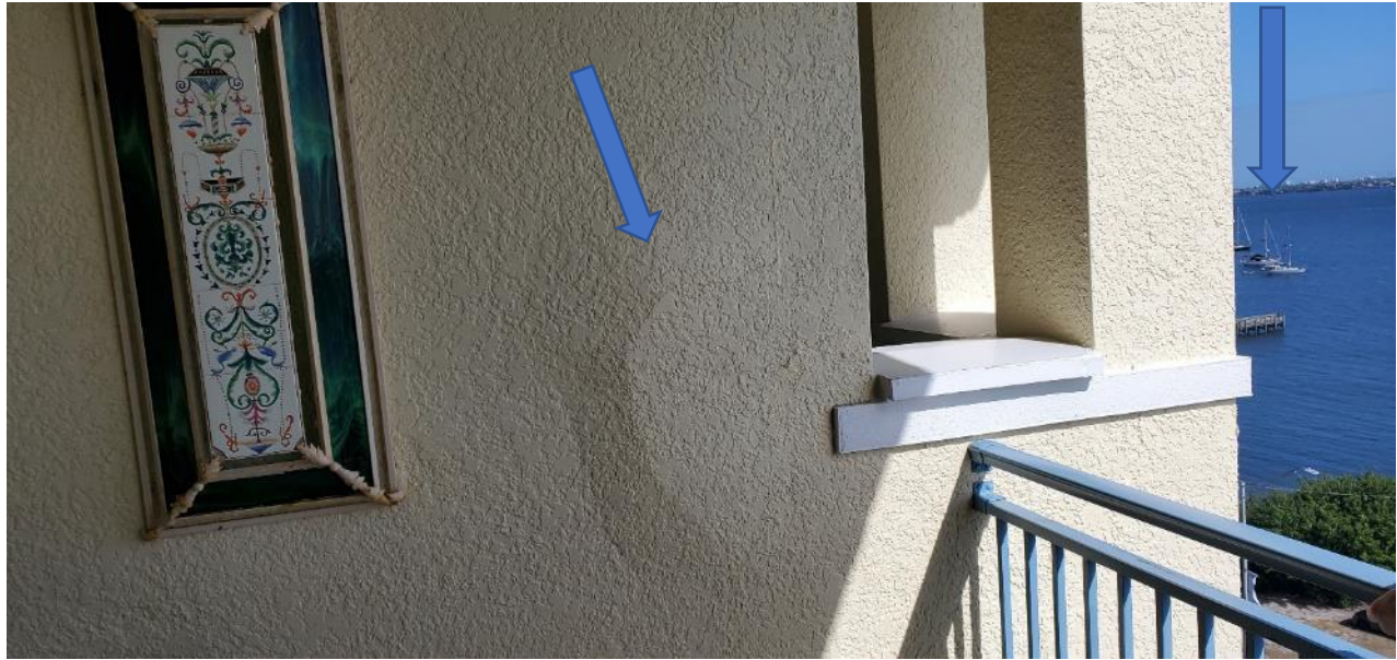
Loose stucco on wall (Unit 801) Repair at next painting cycle
