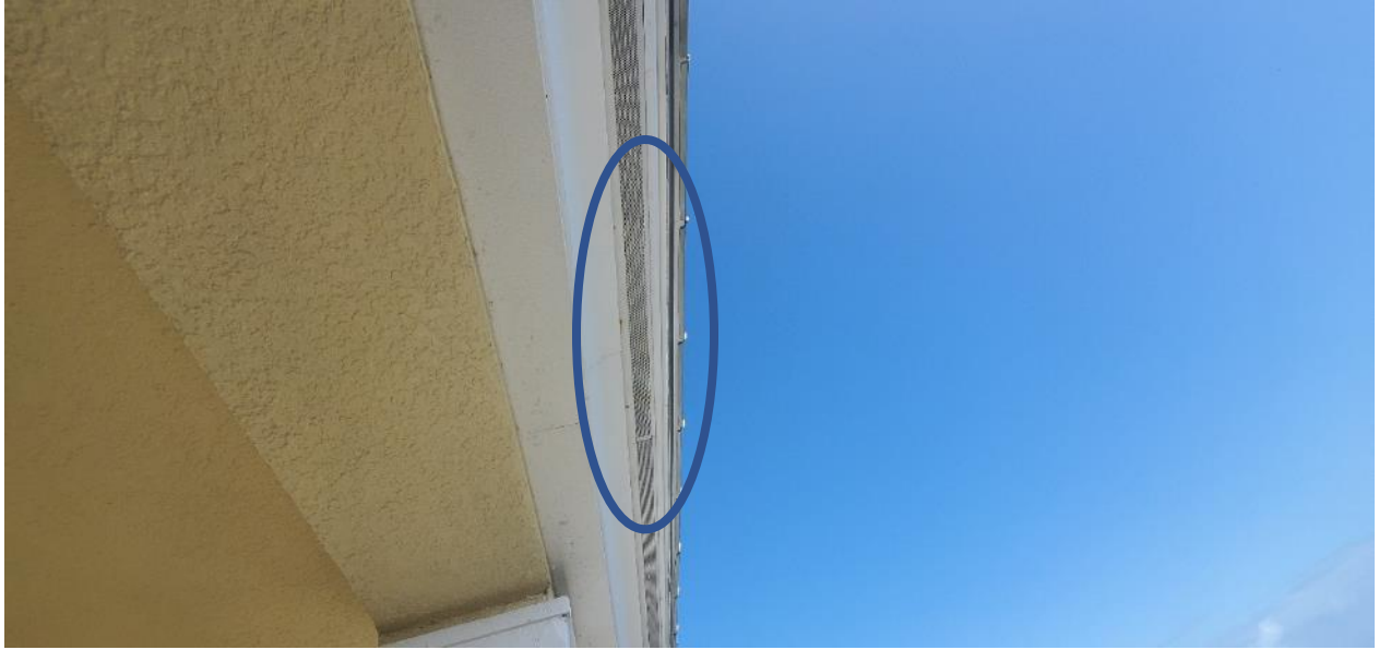
Soffit separation and rust spots (Unit 802)
