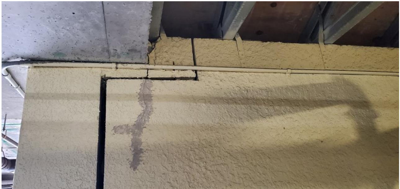
Concrete wall in garage with cracks and spalls Monitor for potential future concrete repair
