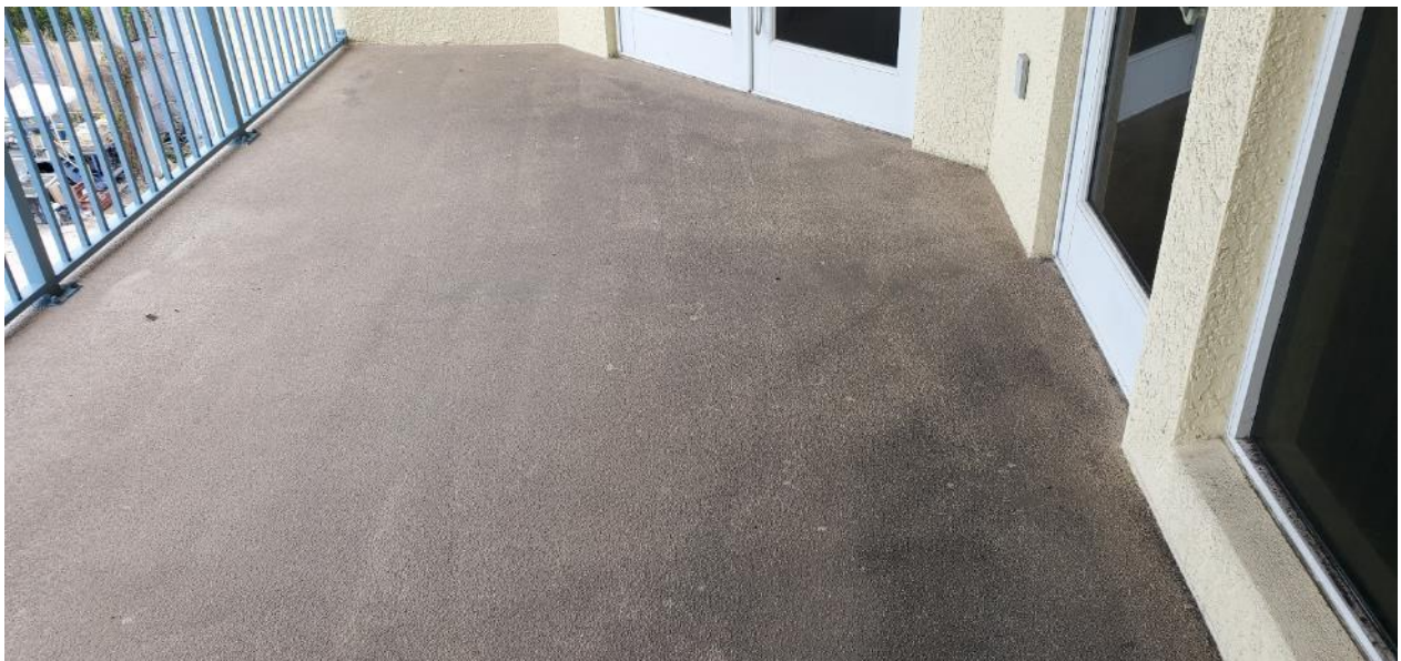
Stained balcony surface. Possible candidate for cleaning and recoating as part of the next painting project. Drainage could be improved during a future restoration project.
