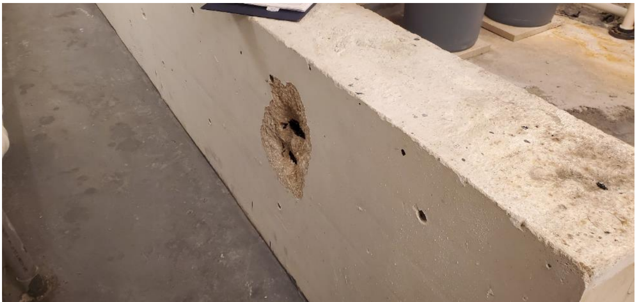
View of spalled knee wall in pool pump room (3 rd Floor) Monitor for potential future concrete repair
