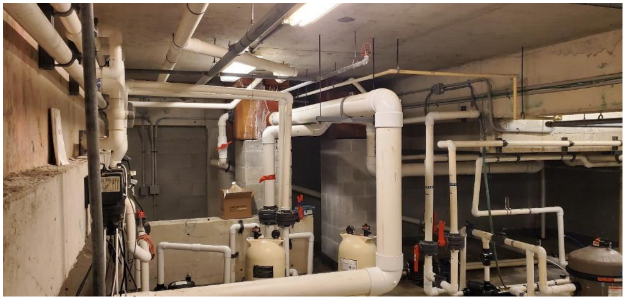
View of pool pump room (3 rd Floor)
