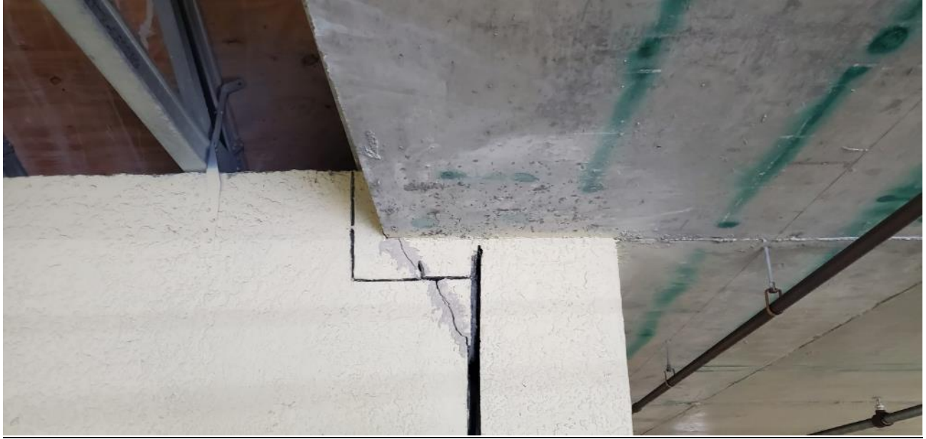
Concrete wall in garage with cracks Monitor for potential future concrete repair
