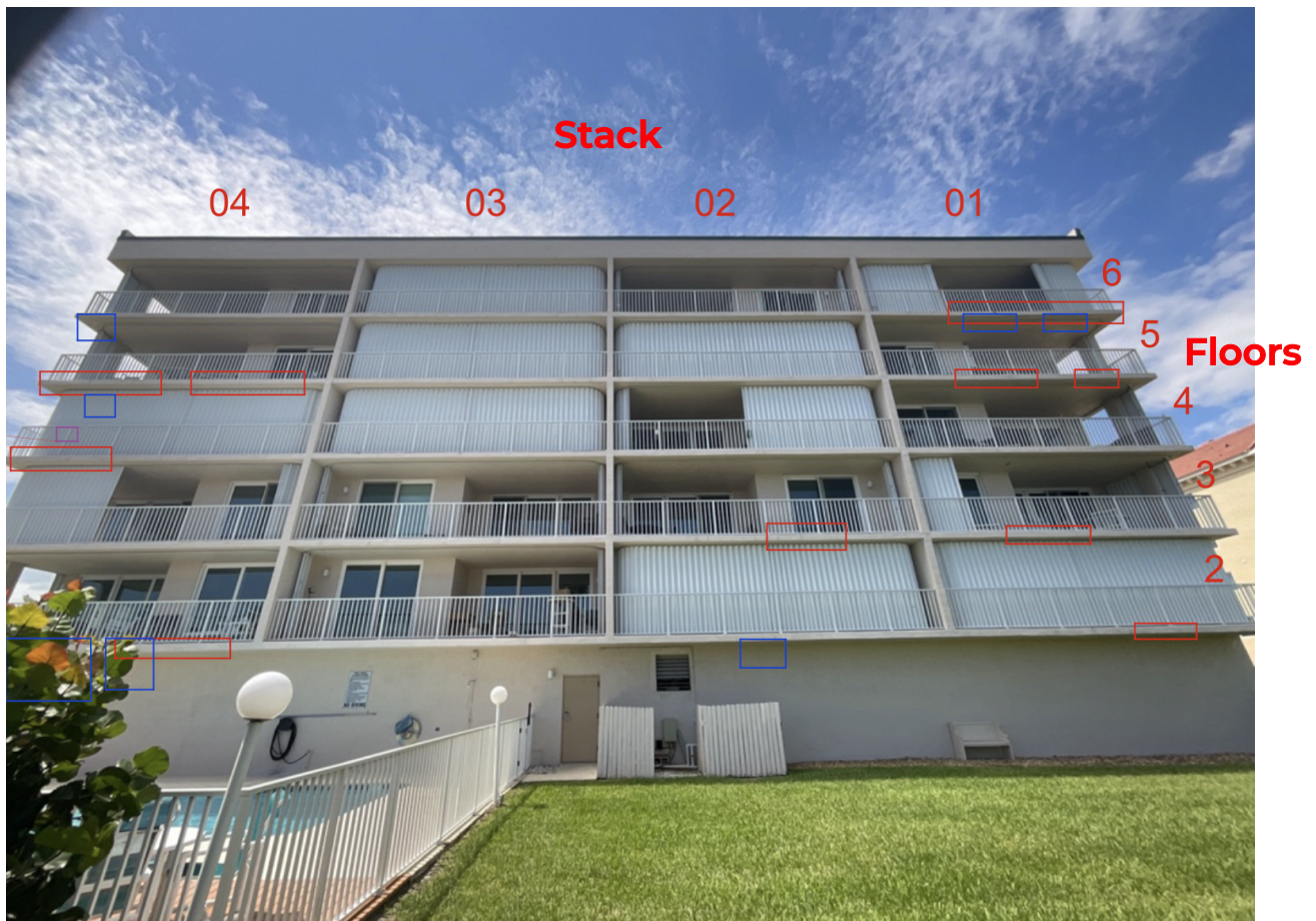
Figure 1. Areas of required remediation based on findings at representative areas during Phase II investigation. Areas in red signify slab edge cracks, areas in blue signify soffit damage, and areas in purple signify column damage.
