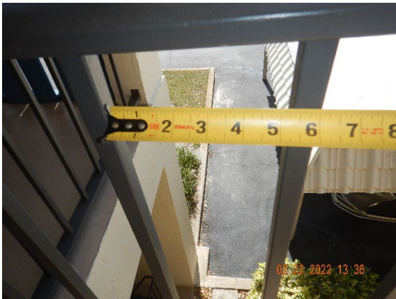
Photograph 7: Excessive rail spacing Not to current building code
