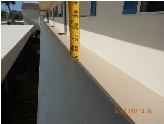
Photograph 5: Aluminum guardrail Not to current building code
