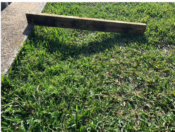
Photograph 15: Straight edge showing washout
