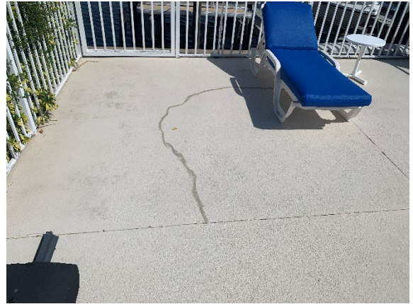
Photograph 16: Pool deck and crack
