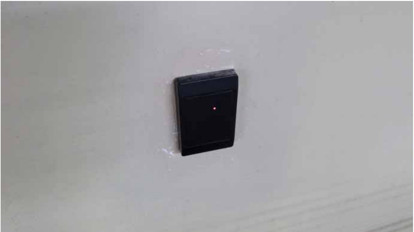
Access Control - FOB Reader
