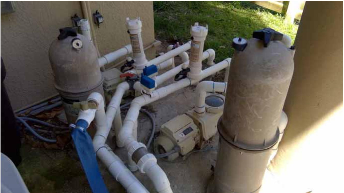
Pool & Spa Equipment
