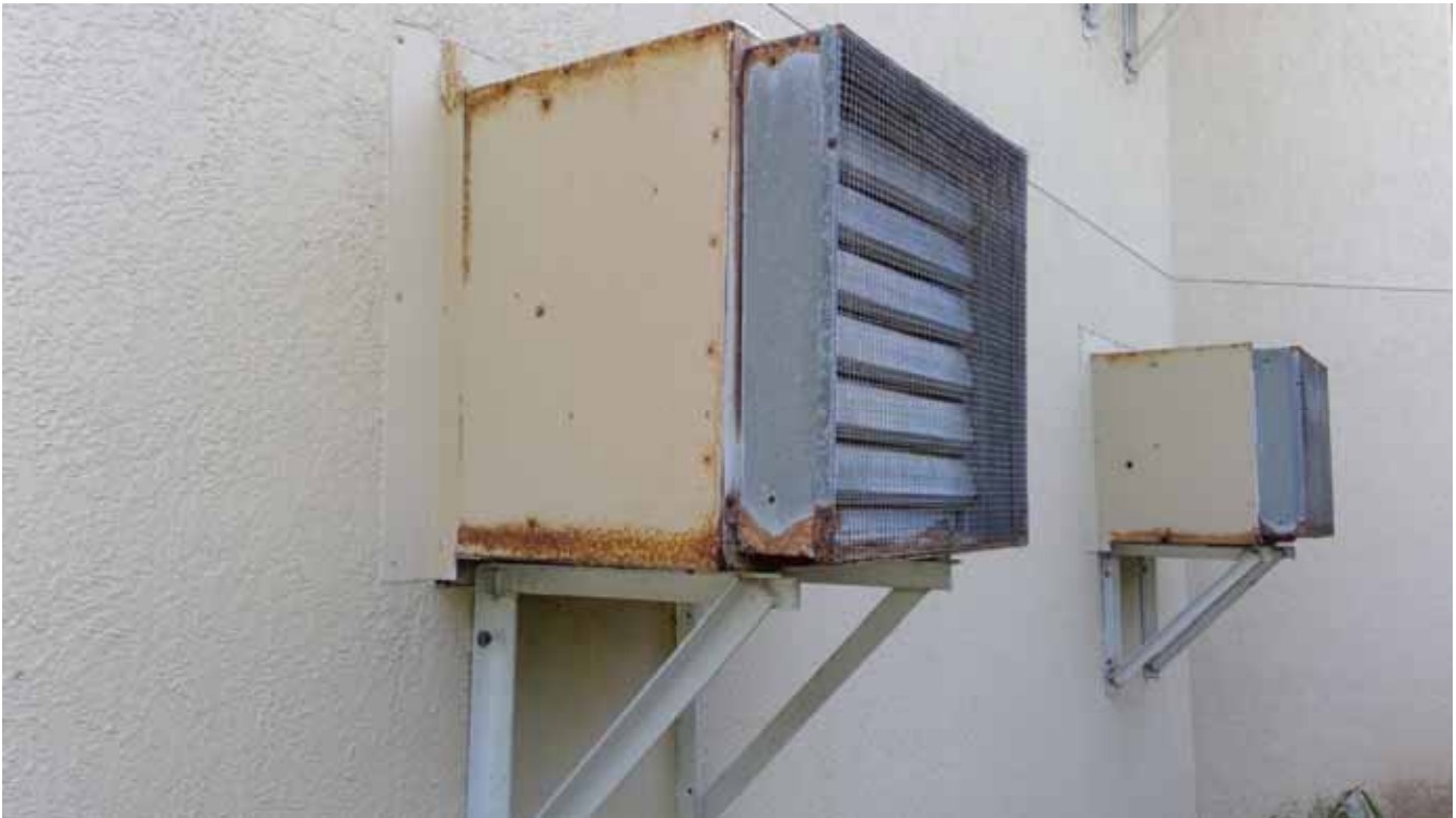
Garage Exhaust Fans
