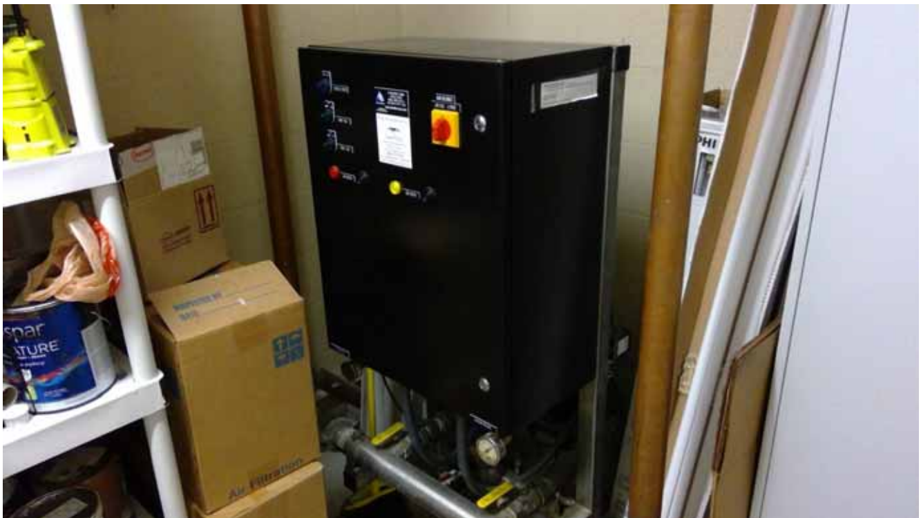
Domestic Water Booster Pump System
