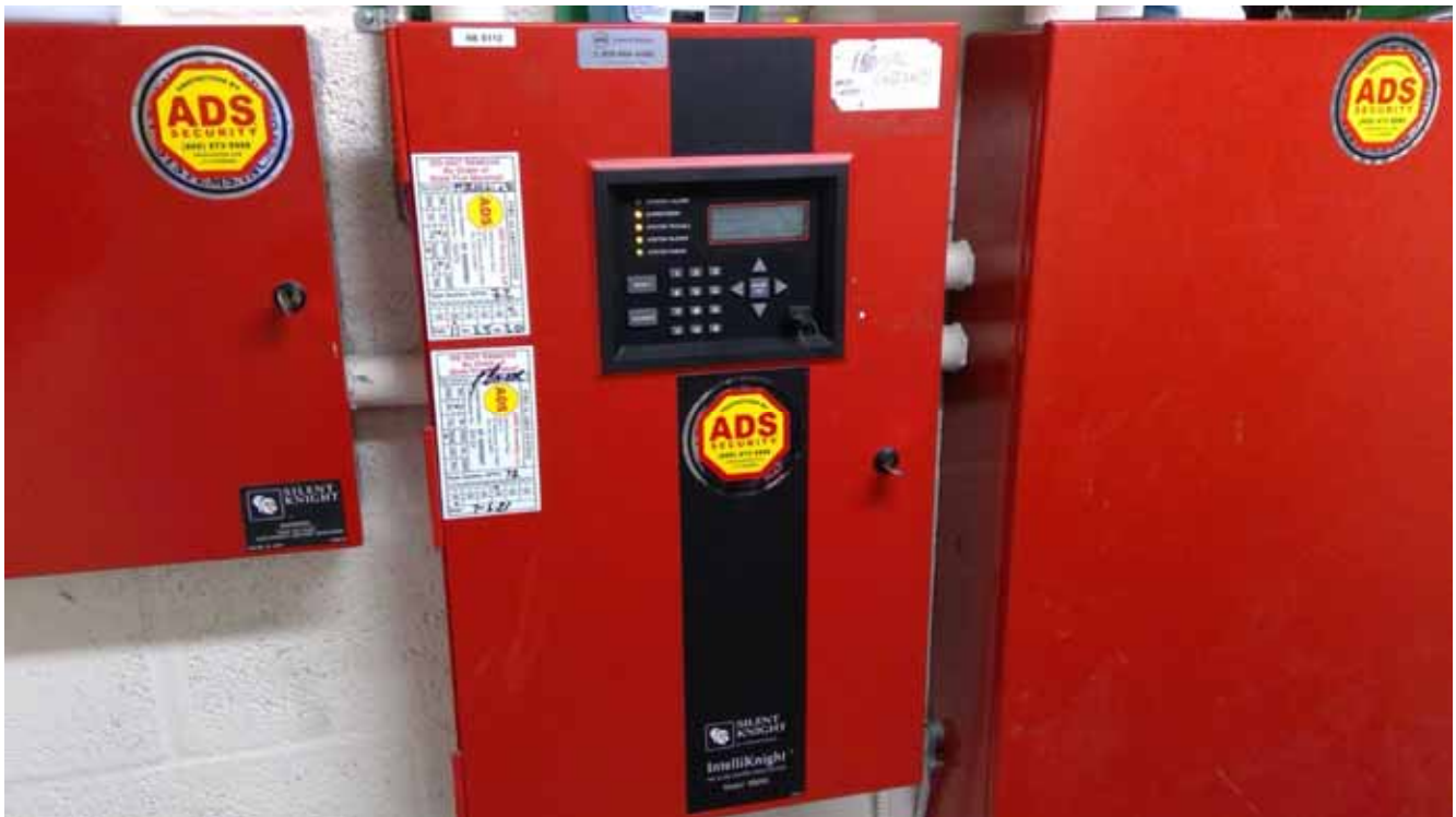
Fire Alarm Panel
