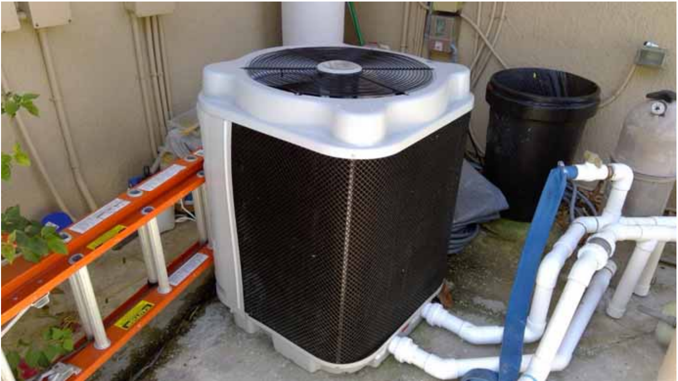
Spa Equipment, Heat Pump
