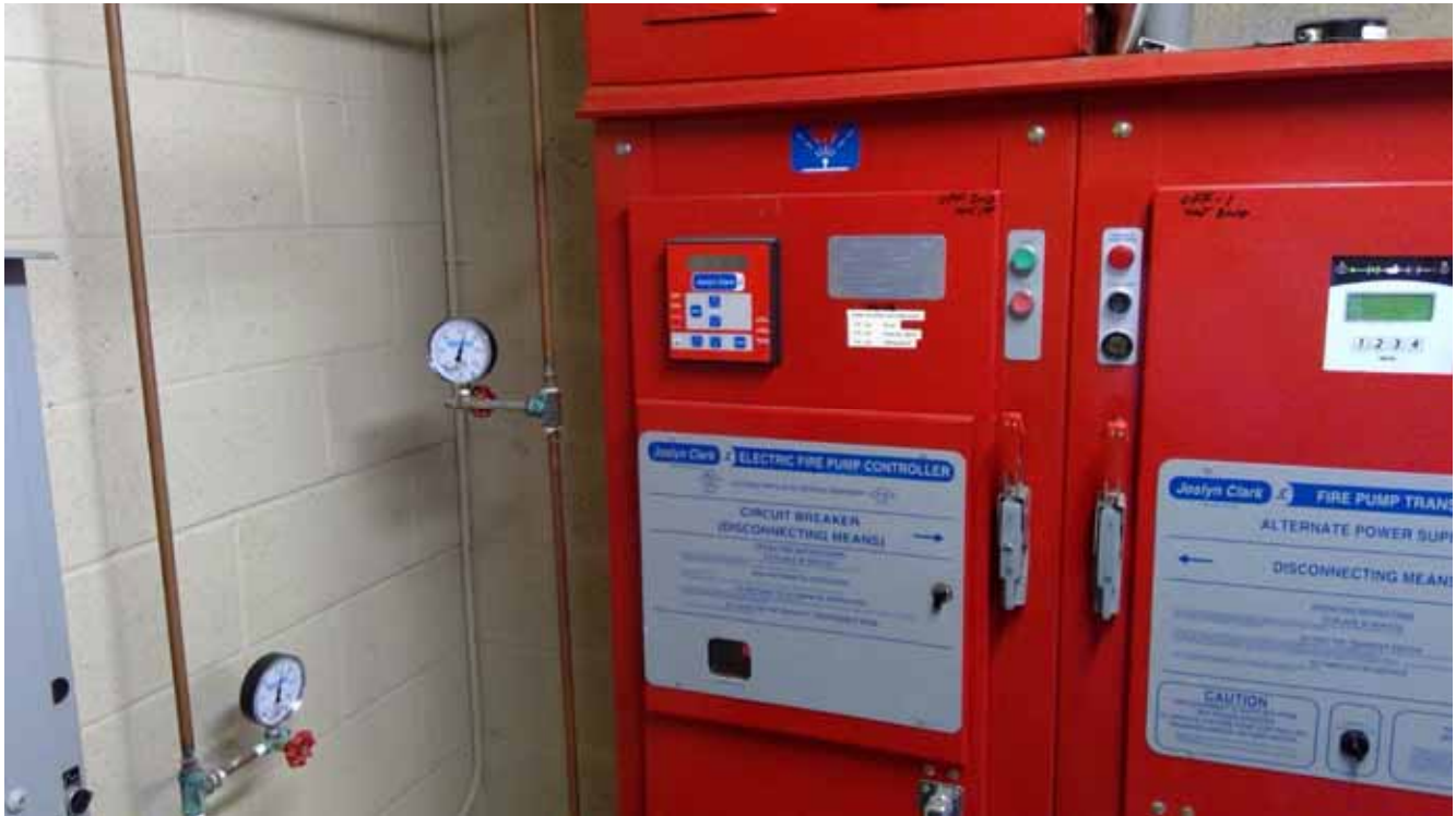
Fire Pump Controller
