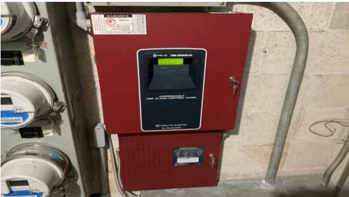
North Condo Bldg Fire Alarm Panel
