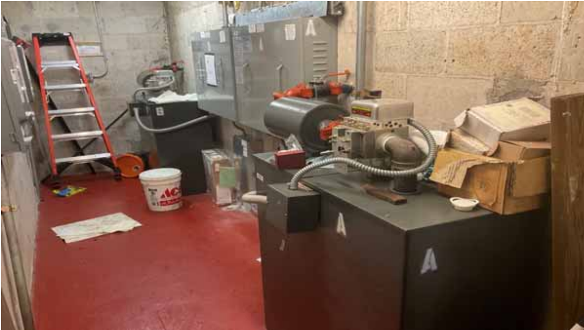
North Condo Bldg Elevator Equipment Rm
