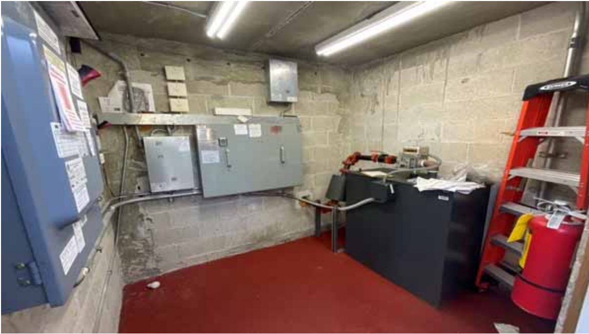
South Condo Bldg Elevator Equipment Rm
