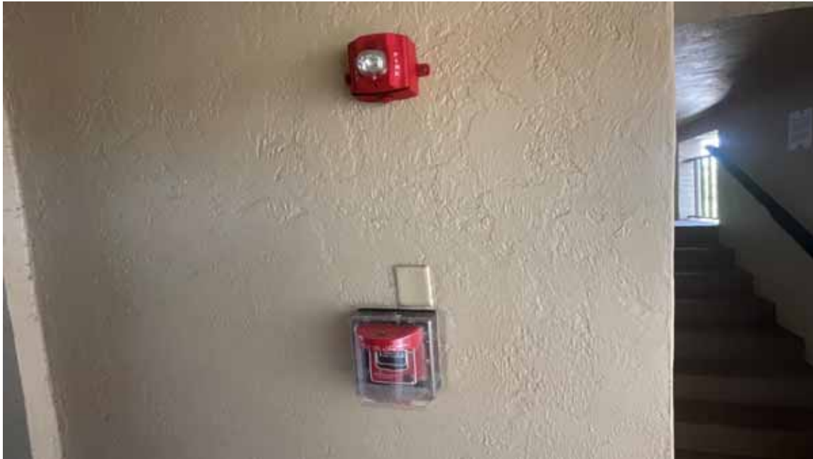
North Condo Bldg Fire Alarm System Devices
