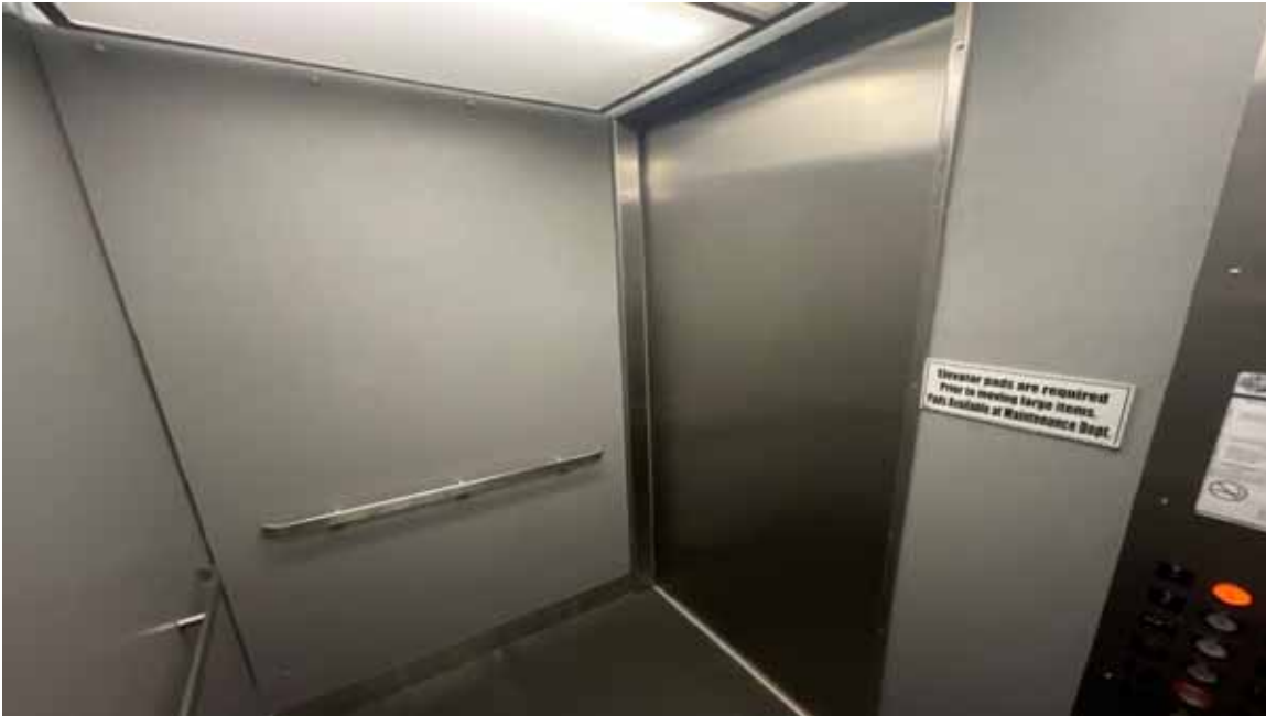
South Condo Bldg Elevator Cab
