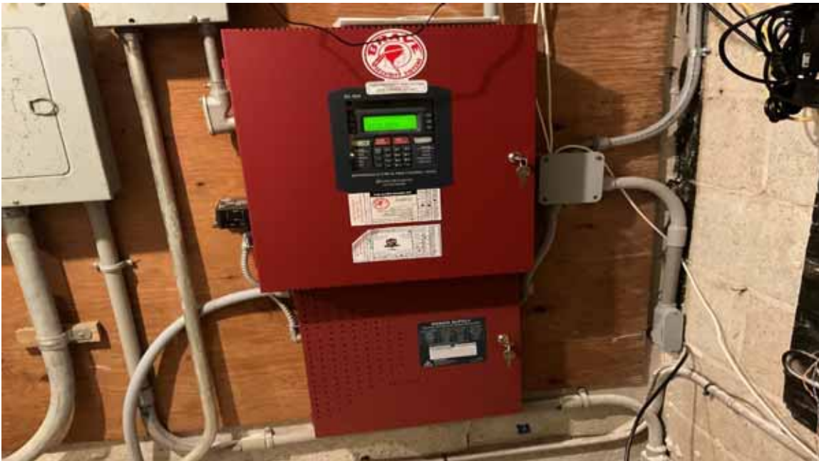
South Condo Bldg Fire Alarm Panel
