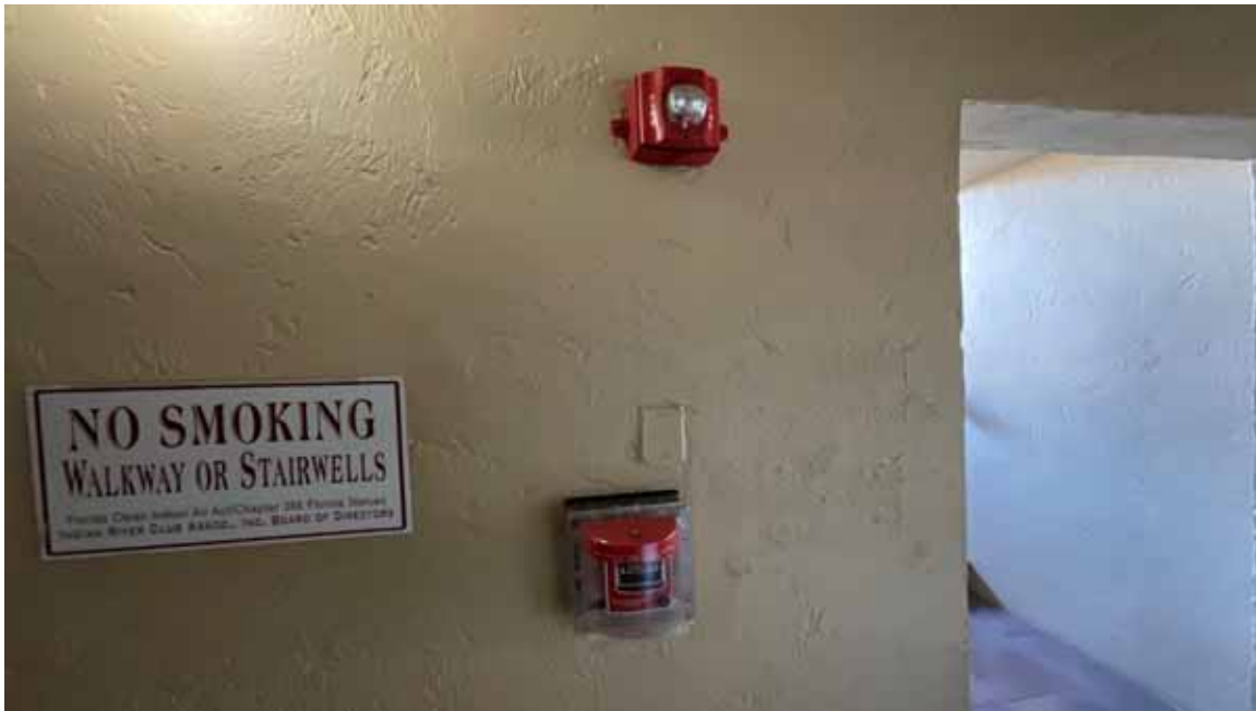
South Condo Bldg Fire Alarm System Devices
