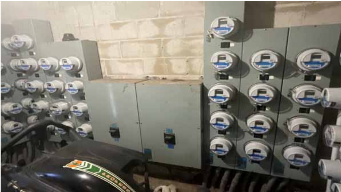
North Condo Bldg Electrical Panels
