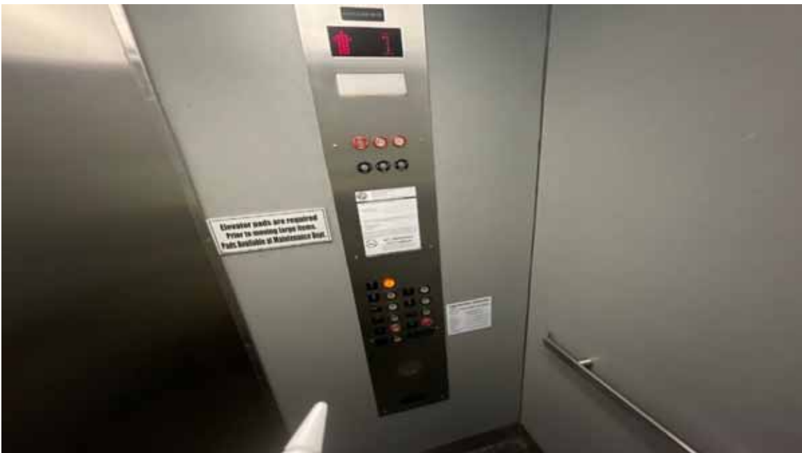
South Condo Bldg Elevator Cab
