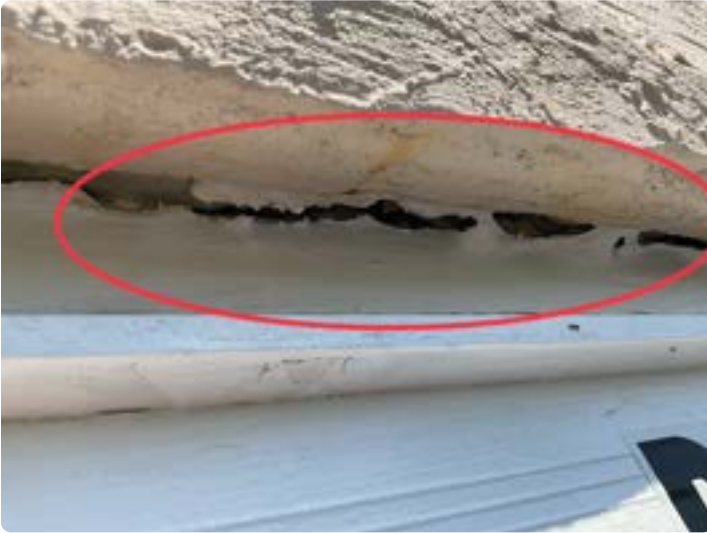
Failed previous remediation above generator room door
