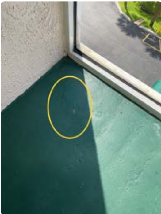
Hollow area near 5th floor elevator
