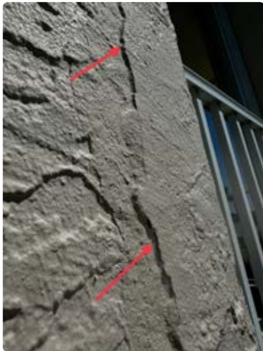
Failed previous remediation on first floor, far-right side of right elevation
