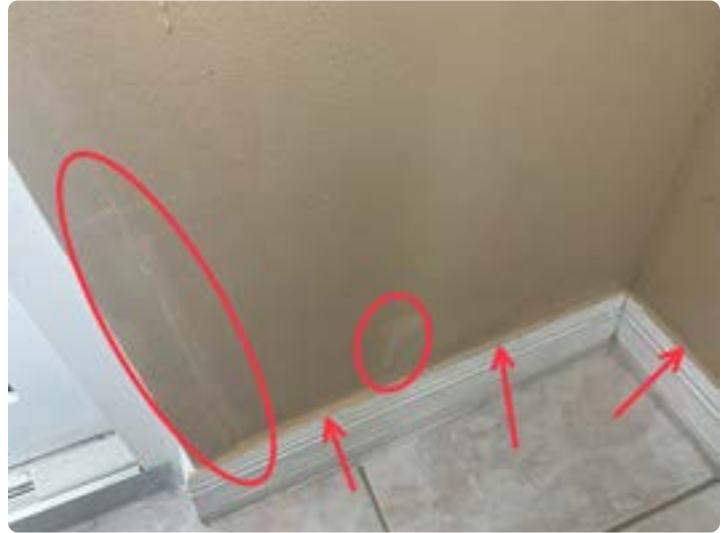
Drywall damage and re-painted area between wall and baseboards in Unit 504
