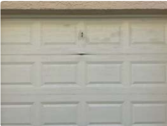
Dent in small garage door
