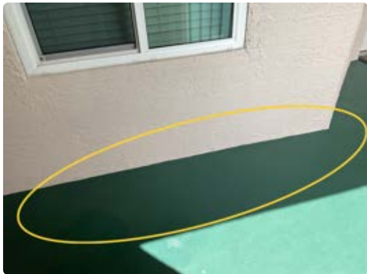
Hollow area near Unit 203
