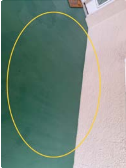
Hollow area near Unit 201. Area has had previous remediation.
