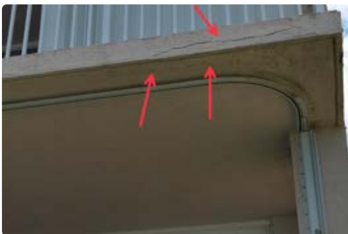
Delaminated coating below crack on Unit 501 balcony slab
