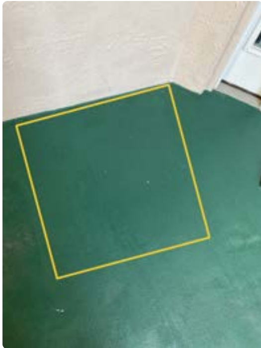
Hollow area on walkway near Unit 504
