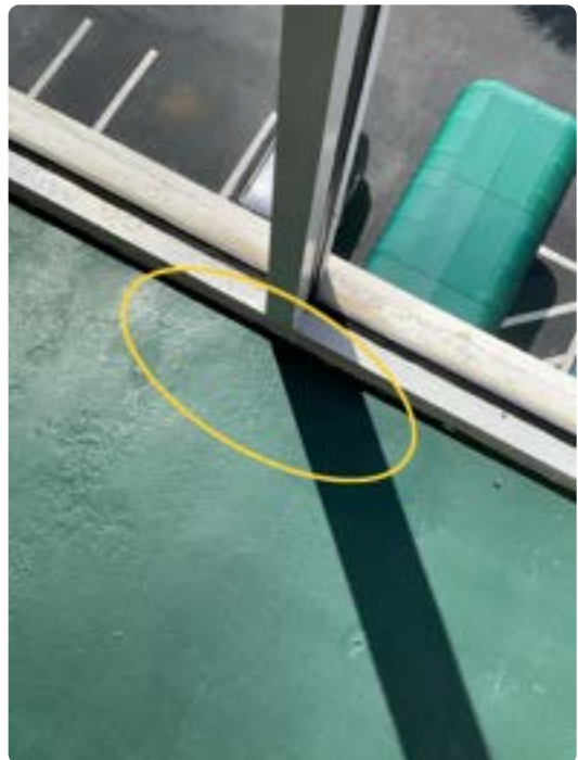
Hollow area near 5th floor elevator
