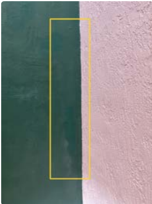
Hollow area near Unit 304
