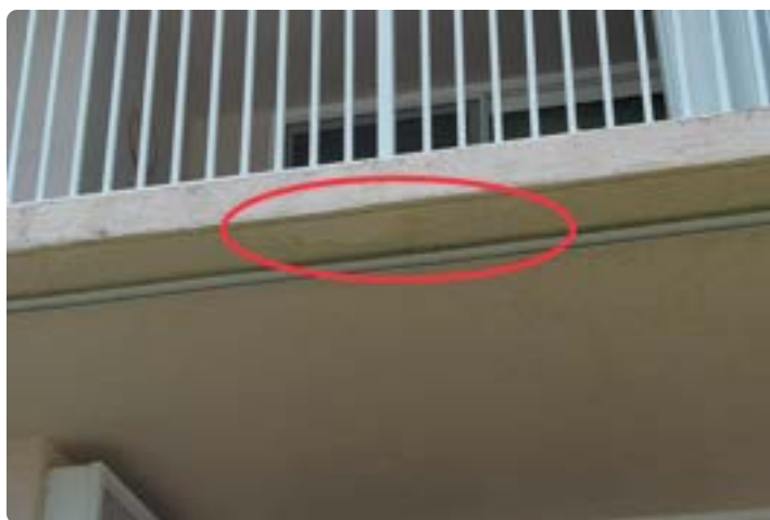
Delaminated coating on Unit 501 balcony slab
