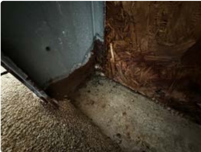
Water damage to sheathing and corroded steel studs due to water intrusion into Unit 304
