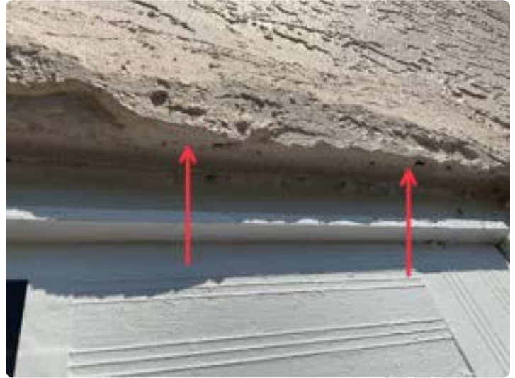
Failed previous remediation above generator room door
