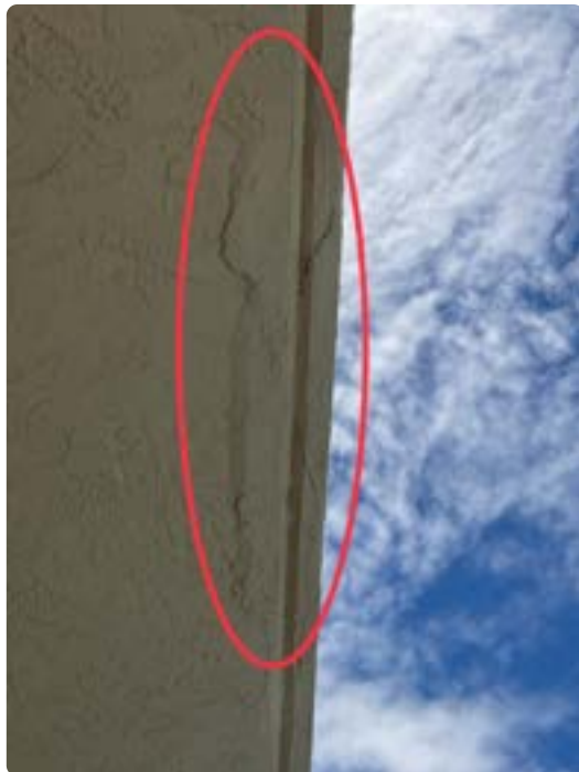
Delaminated stucco and balcony edge spall on Unit 204 balcony
