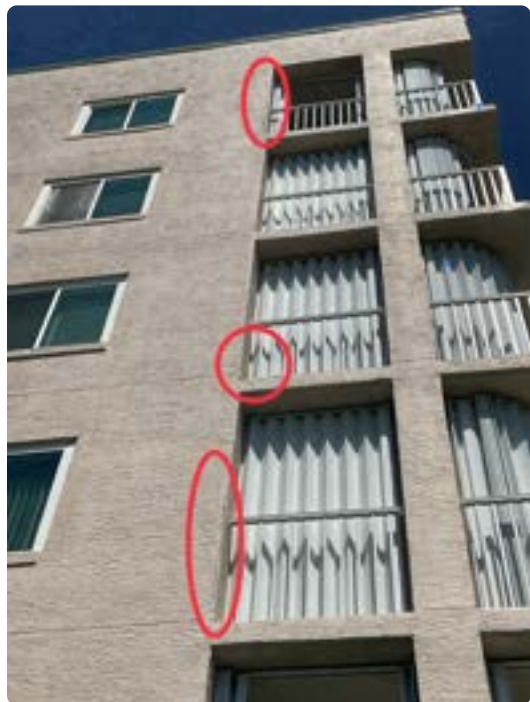
Similar damage identified on 3rd, 4th, and 6th floors on far-right side of right elevation
