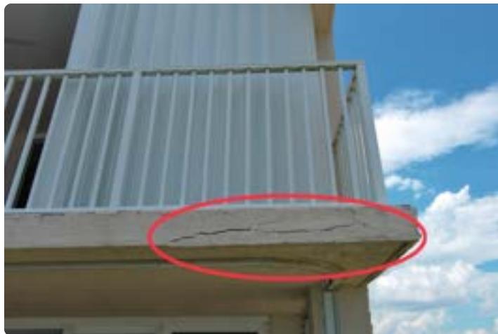
Crack on face of Unit 501 balcony slab
