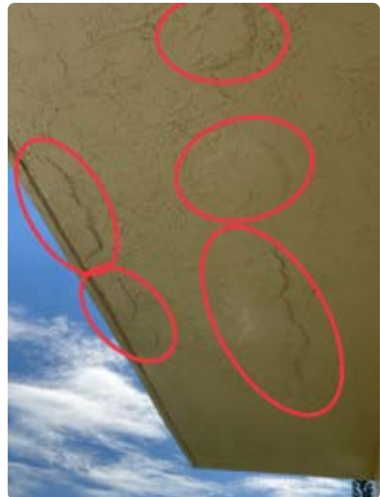
Delaminated coating on Unit 204 balcony
