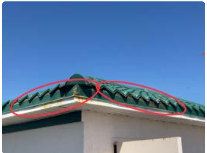
Corrosion on metal roof
