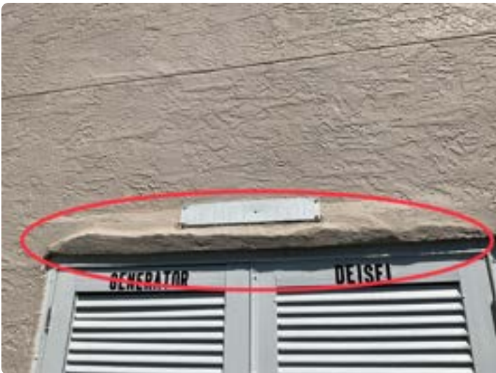
Failed previous remediation above generator room door
