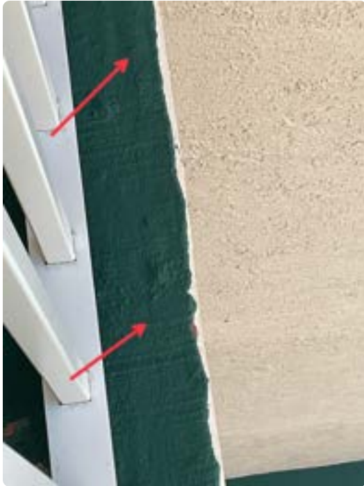
Crack in 5th floor walkway near Unit 502
