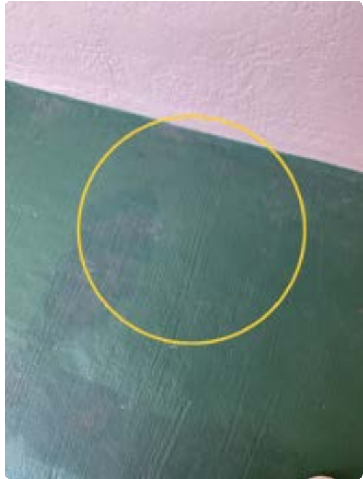
Hollow area near Unit 402. Area appears to have had previous patch.
