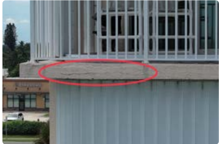
Crack on face of Unit 504 balcony slab
