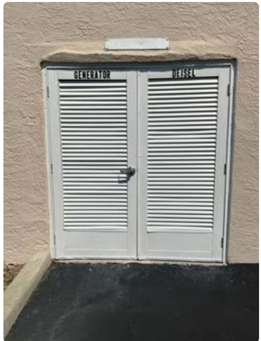
Generator double doors
