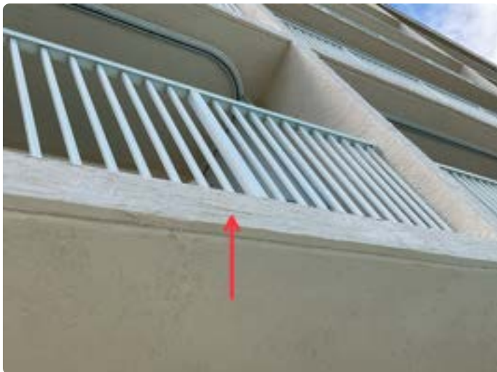
Crack on face of Unit 204 balcony slab
