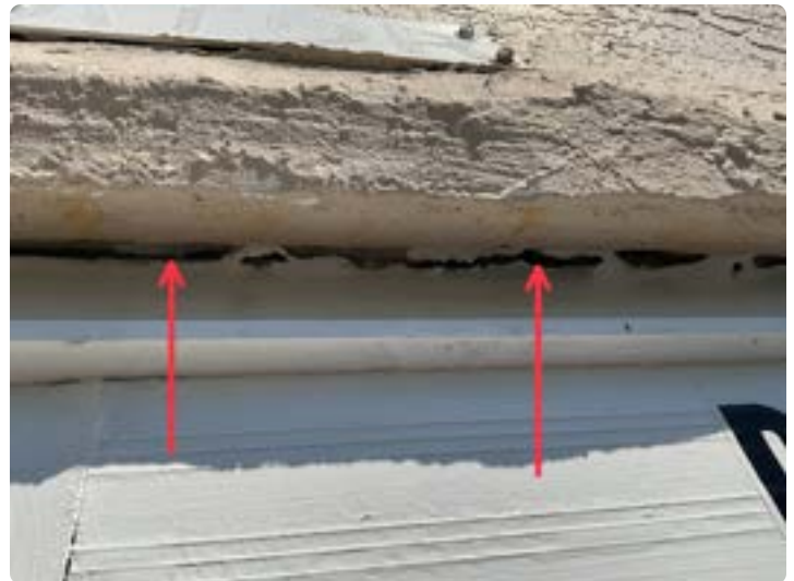
Failed previous remediation above generator room door
