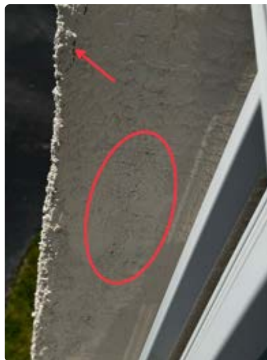
Photo of cracks on third floor from unit balcony
