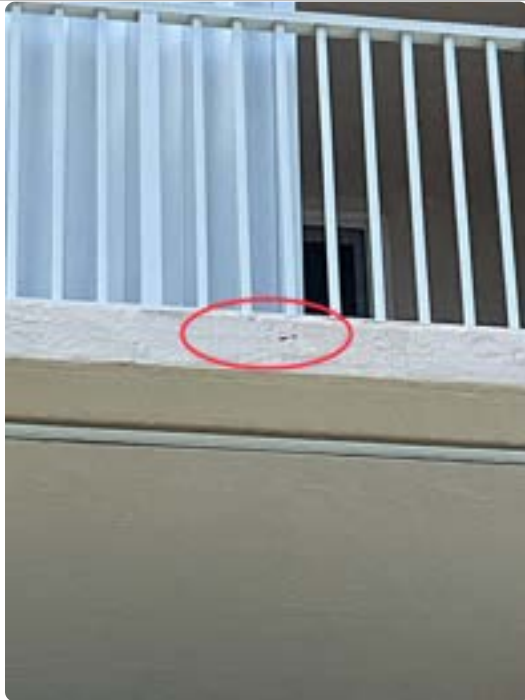
Crack on face of Unit 304 balcony
