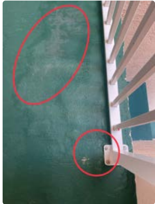
Delaminated walkway paint near Unit 504
