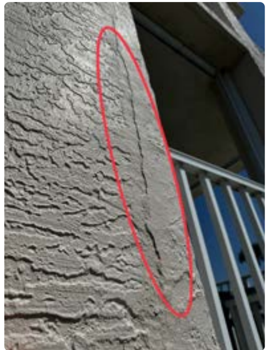
Failed previous remediation on first floor, far-right side of right elevation
