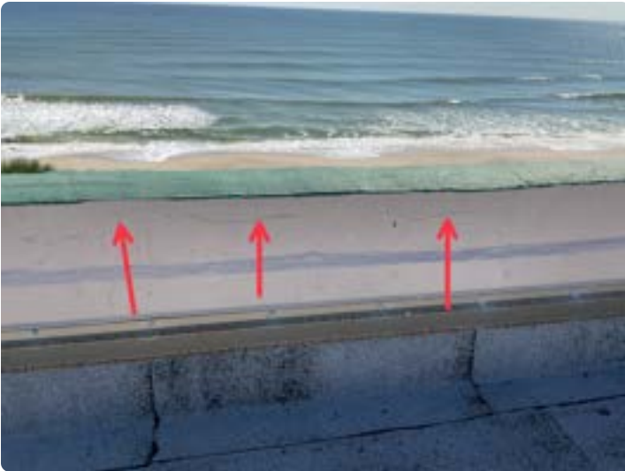
Hairline crack on roof parapet wall
