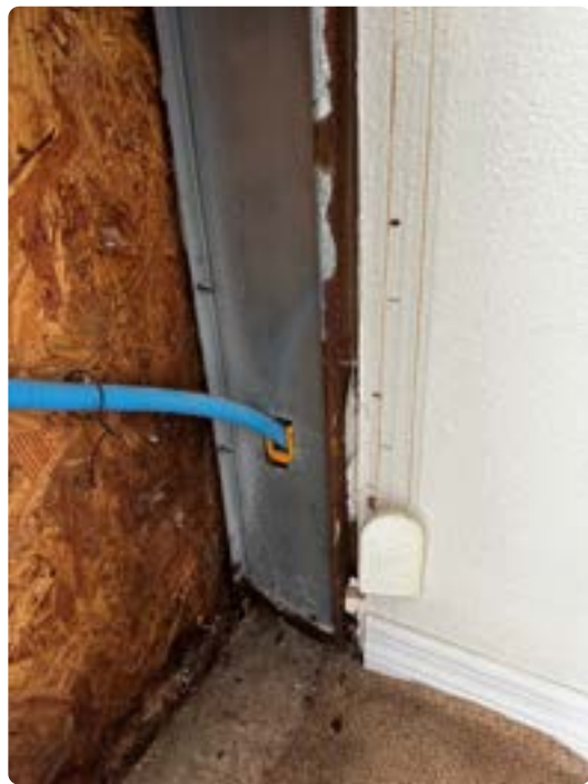
Water damage to sheathing and corroded steel studs due to water intrusion into Unit 304
