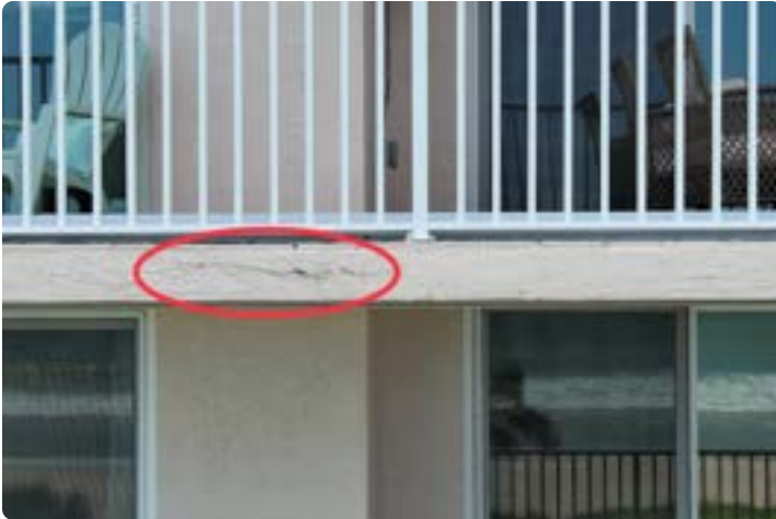
Crack on face of Unit 401 balcony slab
