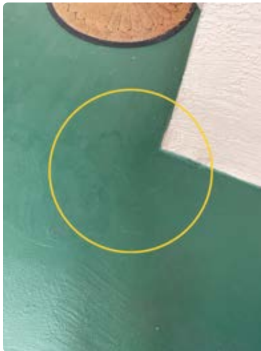
Hollow area near Unit 203
