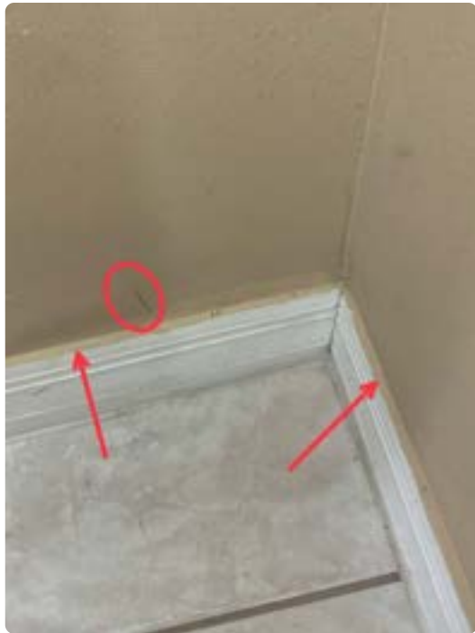
Drywall damage and re-painted area between wall and baseboards in Unit 504
