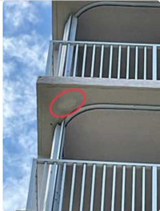
Painted over rust spot on Unit 504 balcony
