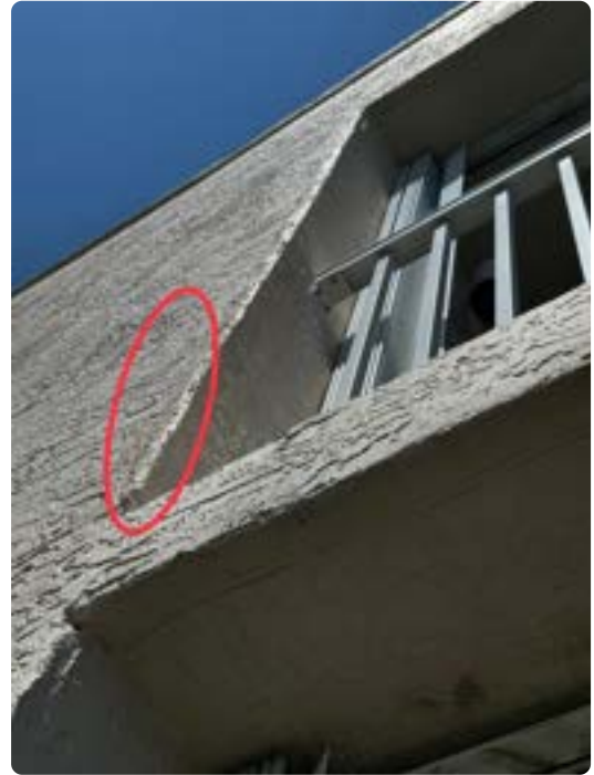
Photo of cracks on 6th floor from 5th floor balcony
