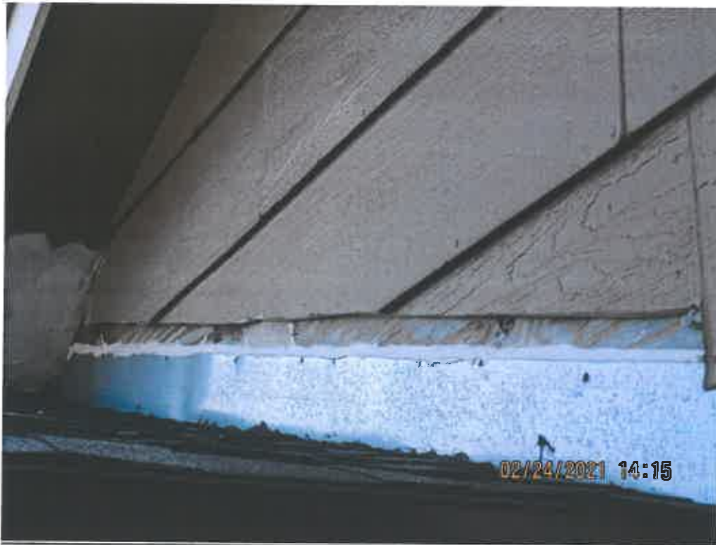
Example view of exposed plywood substrate at recently installed roof flashing-these details and overall poor condition of siding will necessitate siding replacement
