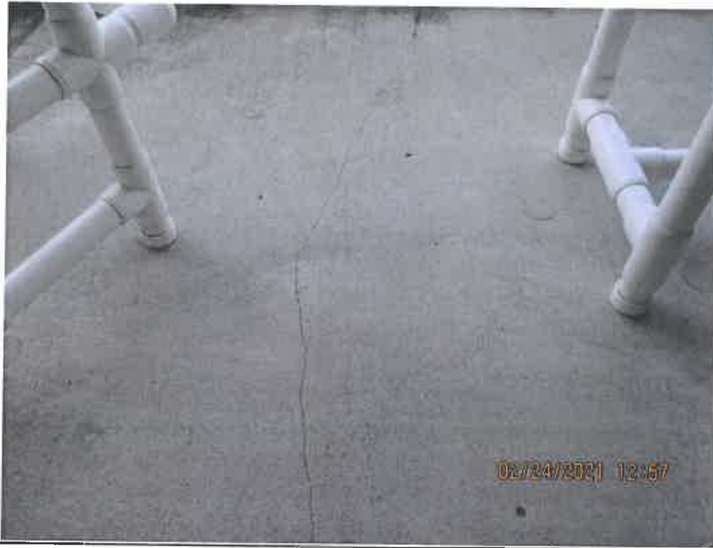
Example view of balcony slab cracks due to lack of proper waterproof coatings-that will lead to concrete spalling and support wood rot
