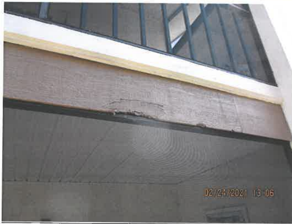
Example view of rotted wood fascia
