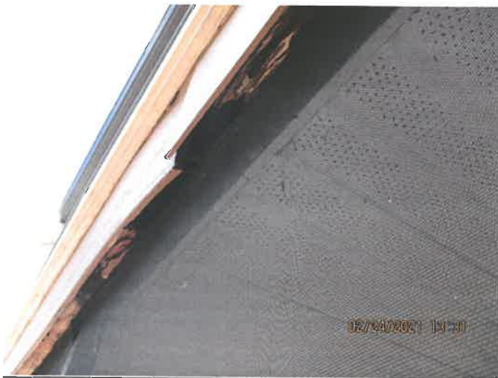
Example view of rotted wood fascia
