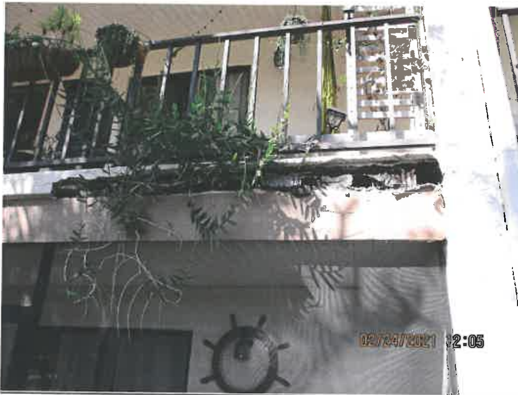
Example view of balcony slab edge failure (unit 106) and exposed wood support framing
