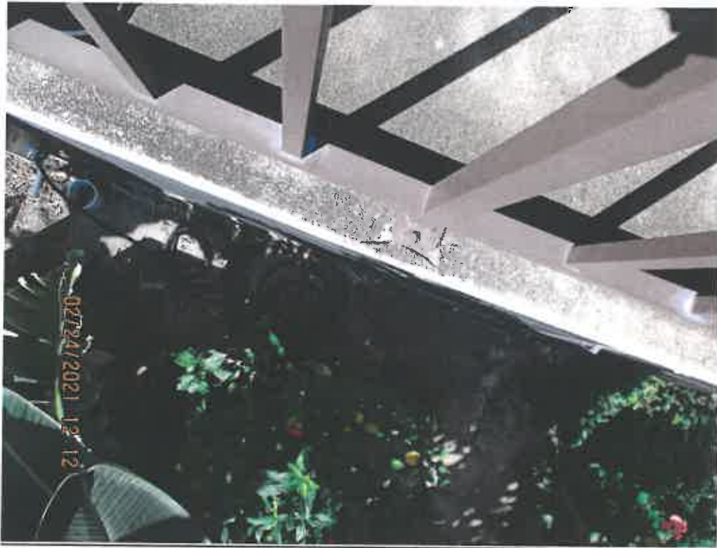
Example view of unsealed railing fastener installation that will lead to water intrusion, concrete spalling and rotted wood
