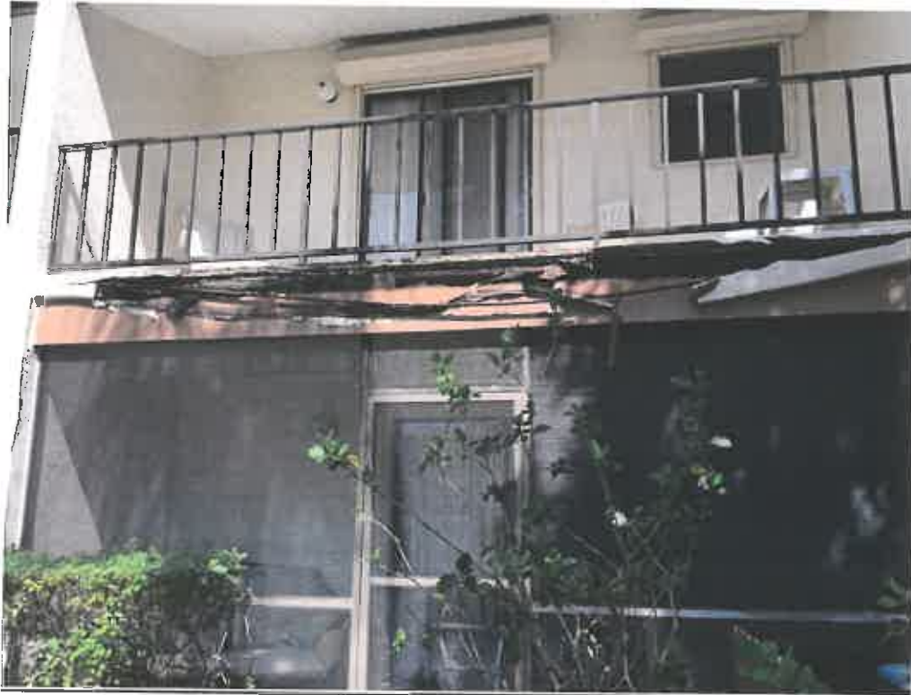
Example view of past balcony edge damage (unit 104) reportedly repaired in 2016
