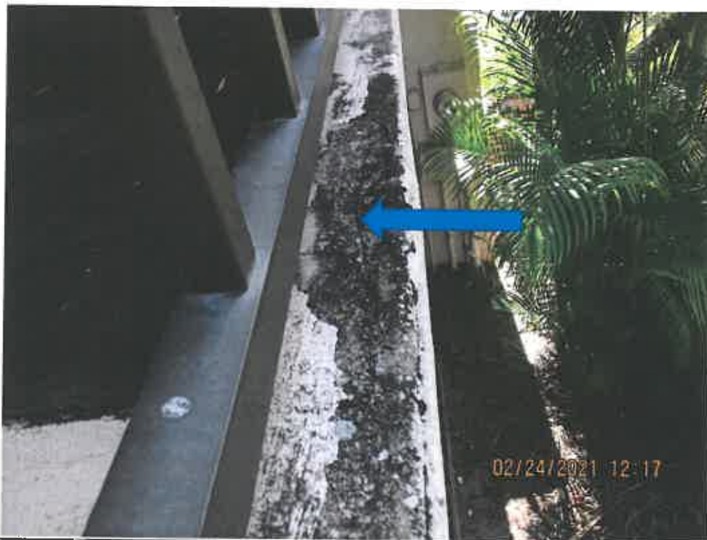
Example view of balcony slab cracks (edge spalling) due to lack of proper waterproof coatings-that will lead to concrete spalling and support wood rot
