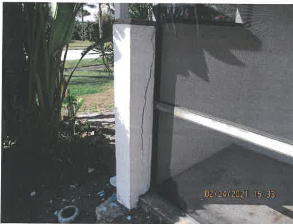
Example view of wing end wall failure due to soil settlement and erosion or spalling
