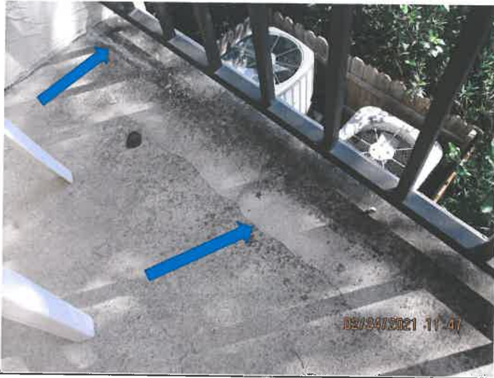
Example view of balcony edge cracking indicative of slab edge spalling due to reinforcing steel corrosion
