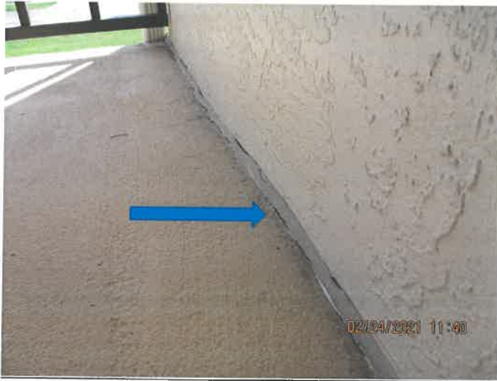
Example view of failing floor to wall sealant-will lead to concrete spalling and wood rot due to water intrusion
