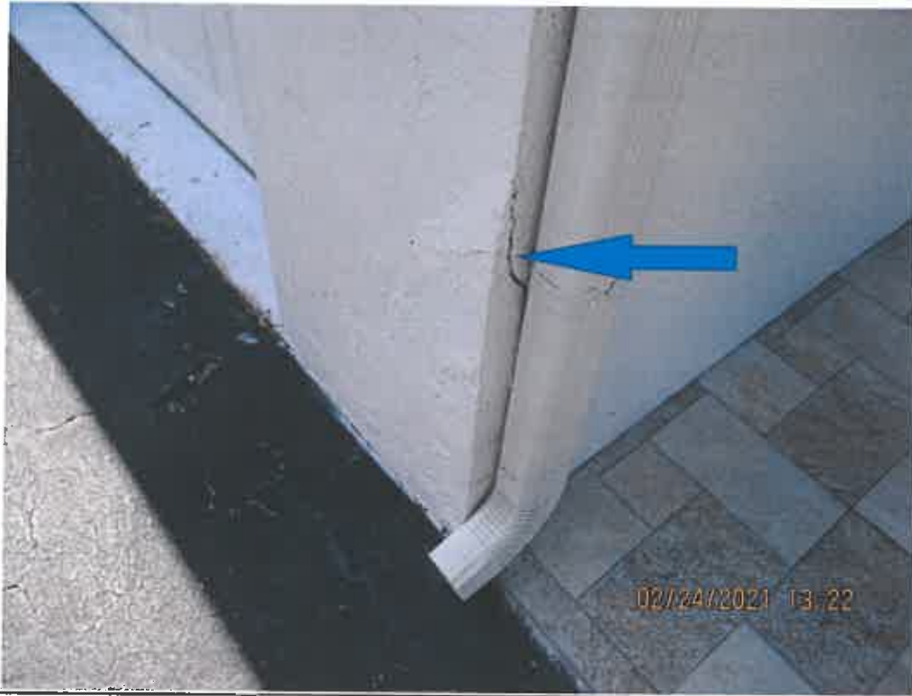
Example view of garage column cracking and spalling due to reinforcing steel corrosion
