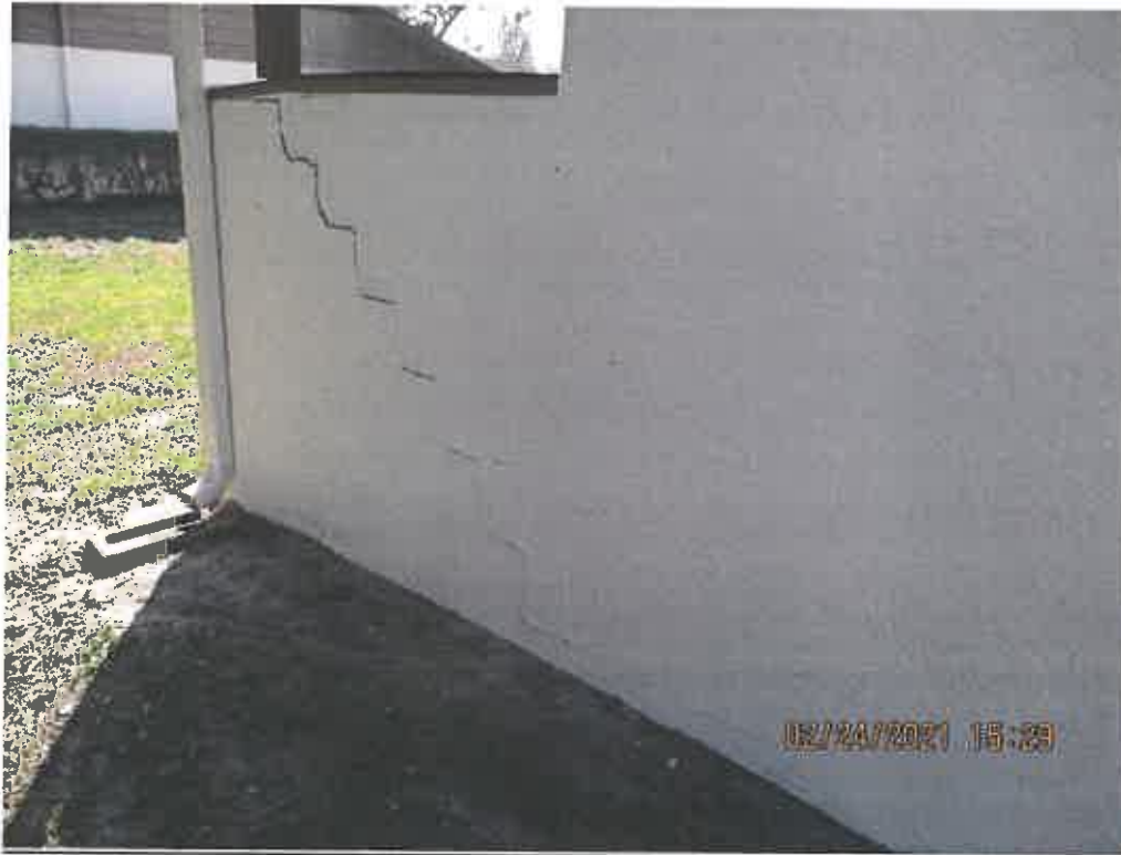
Example view of wing end wall failure due to soil settlement and erosion
