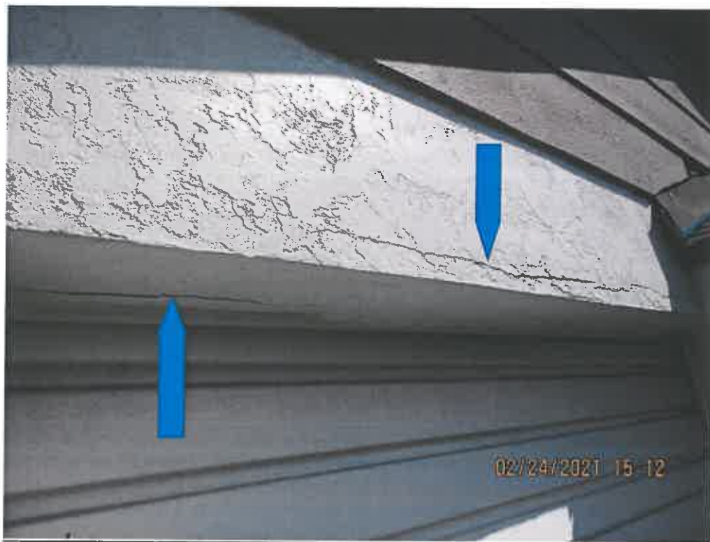
Example view of garage header beam cracking and spalling due to reinforcing steel corrosion
