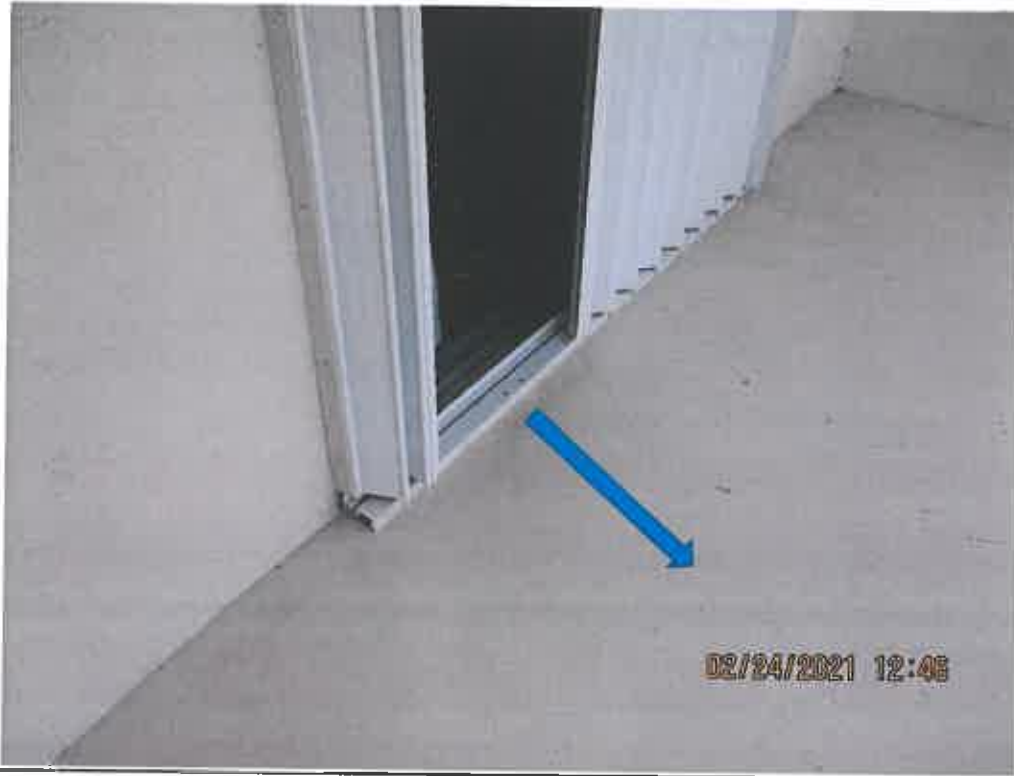
Example view of shutter track installed without recommended drainage shims-will lead to concrete spalling and wood rot due to lack of positive drainage away from door
