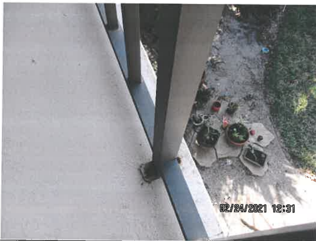
Example view of unsealed corroding railing fastener installation that will lead to water intrusion, concrete spalling and rotted wood
