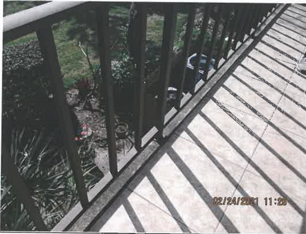
Example view of tiled balcony slab which provides a lack of proper waterproofing-that will lead to concrete spalling and support wood rot
