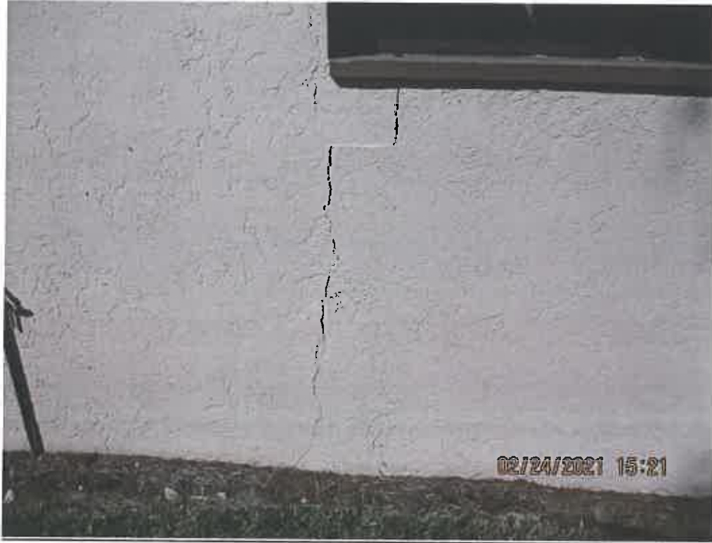
Example view of stucco wall cracks that can allow water intrusion-solved with a proper painting and waterproofing process
