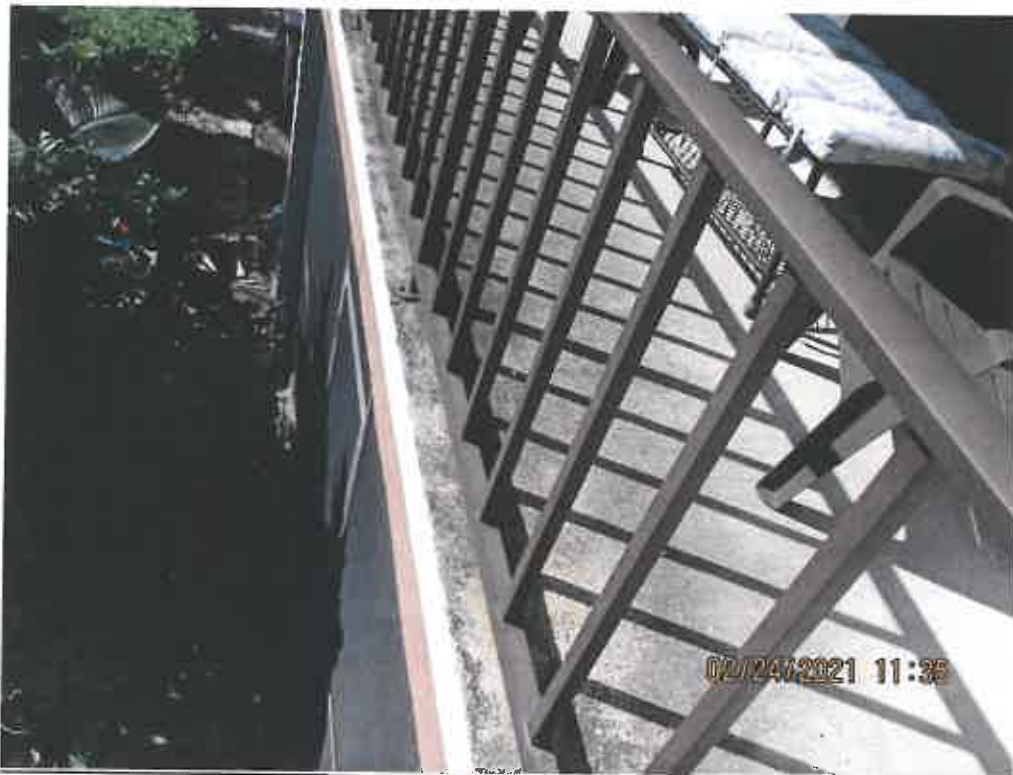
Example view of balcony slab with lack of proper waterproof coatings-that will lead to concrete spalling and support wood rot
