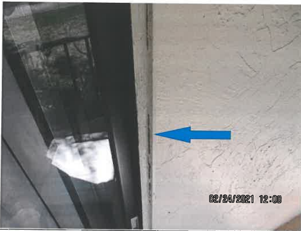
Example view of failing door perimeter sealant-will lead to concrete spalling and wood rot due to water intrusion
