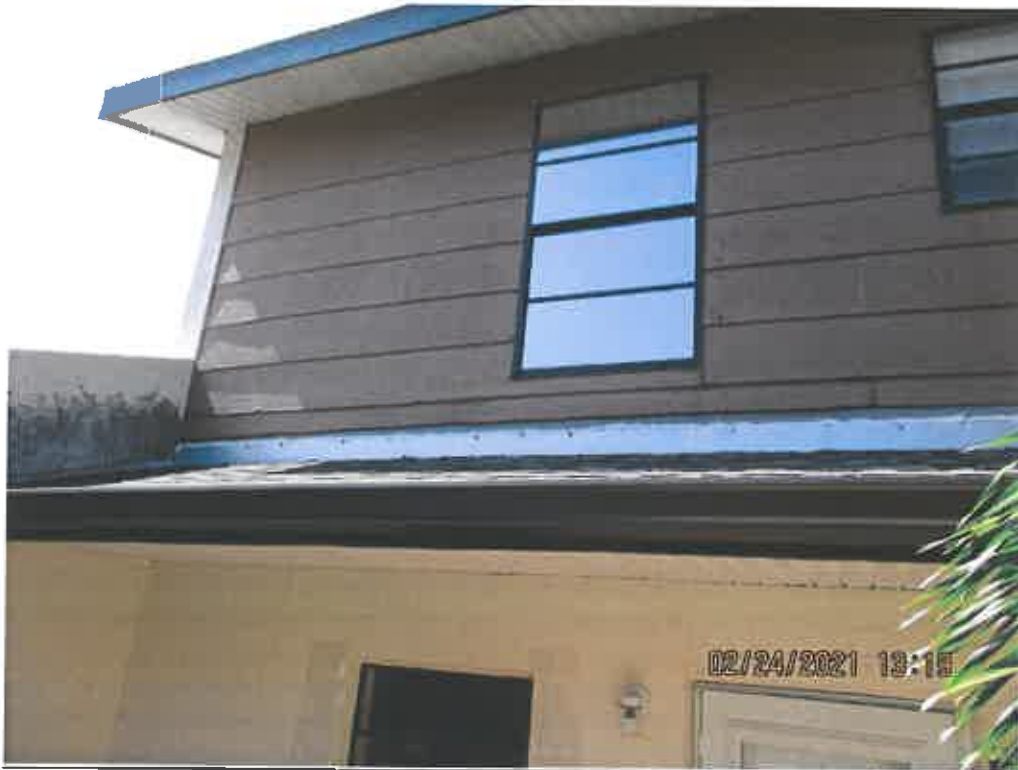
Example view of exposed plywood substrate at recently installed roof flashing-these details and overall poor condition of siding will necessitate siding replacement
